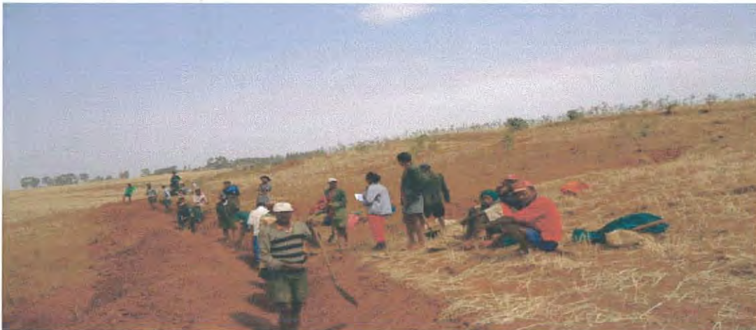
Figure 10: Construction of cut off drain during field observation (own photo at the field)
