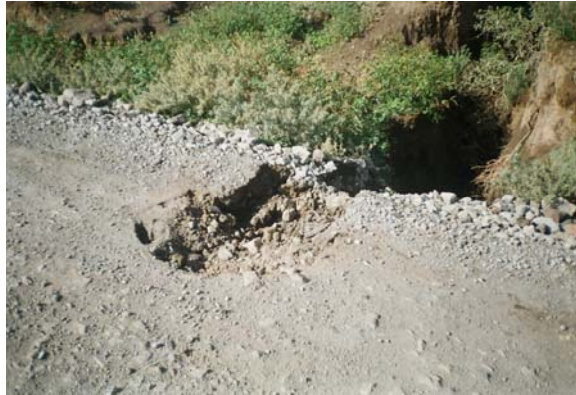
Figure 4.5 Re-collapsing of filled road crack ,Ziway-Butajira (Adopted from: Kebede Mideksa, 2007)
