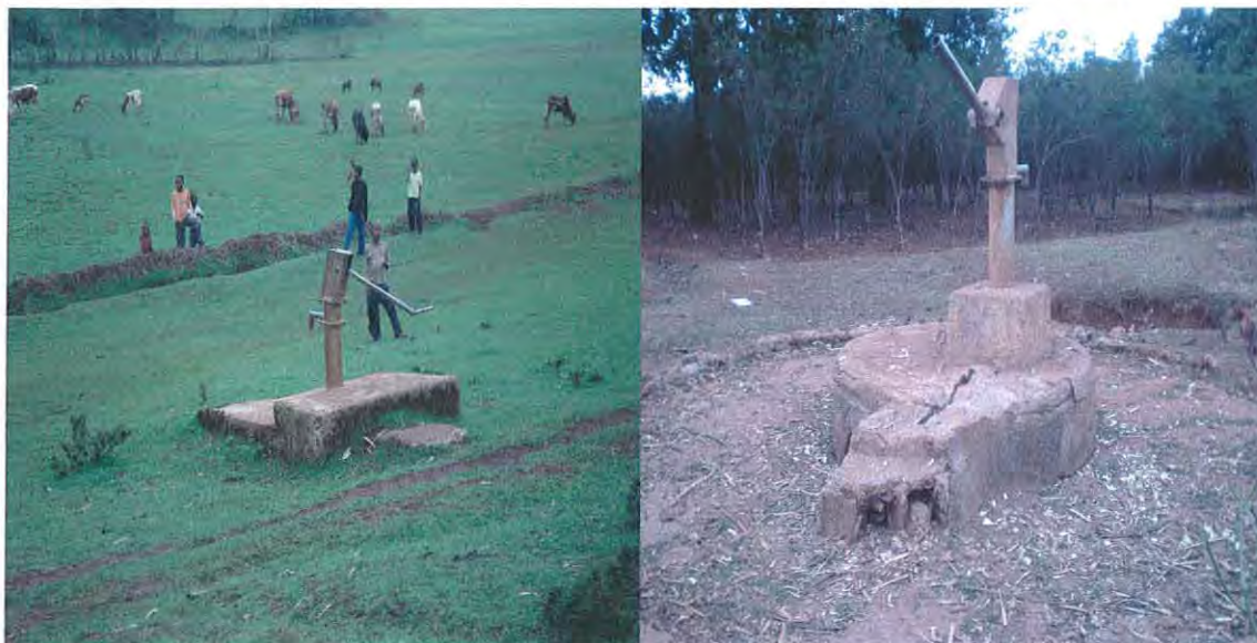
Figure 4.6. Handpump located on marshy ground (left), top work cracked HP(right)
