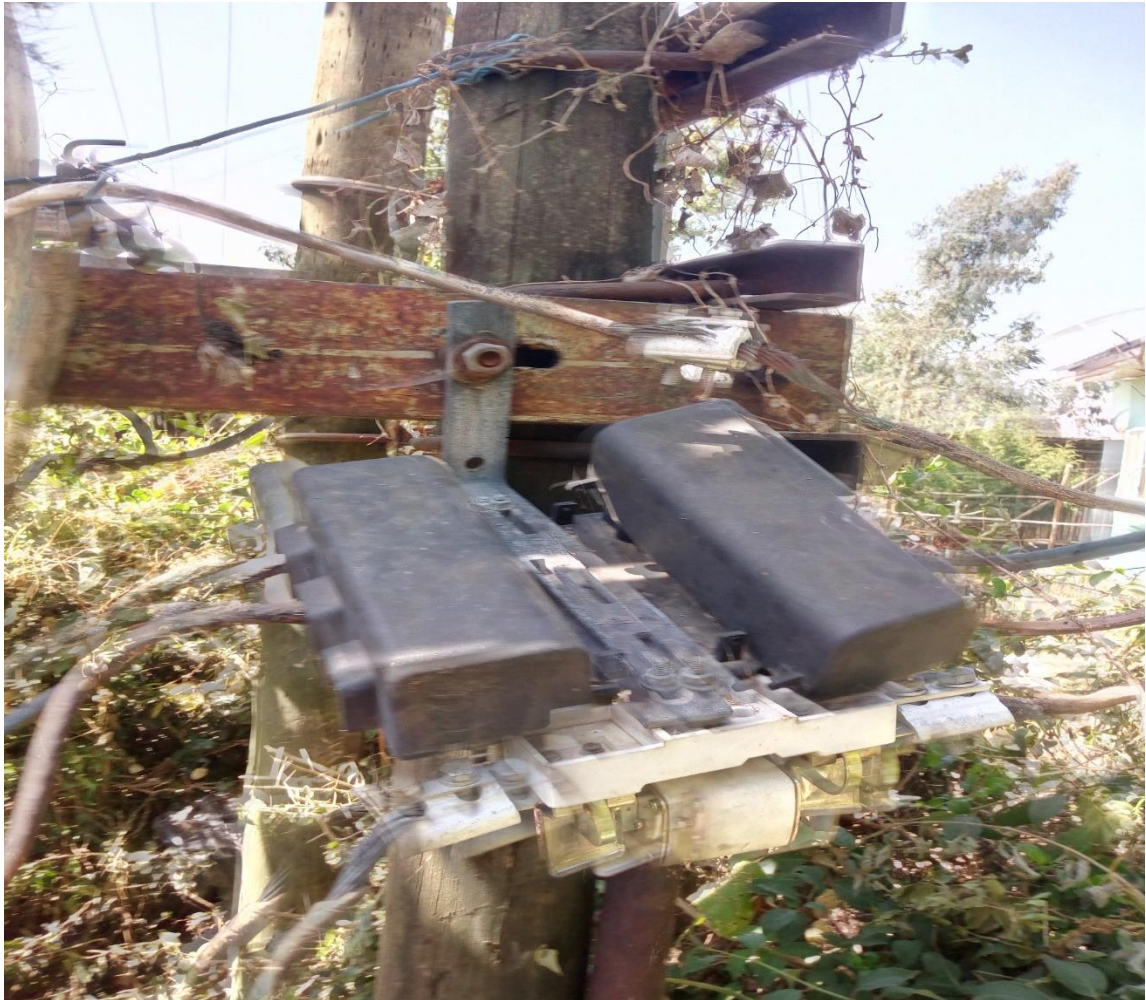
Figure 3. 1 Photo taken by the authors to show aged line connections
