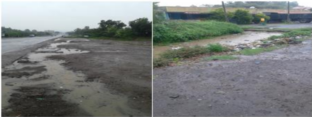
Figure 1-1 The drainage system problems on infrastructures
