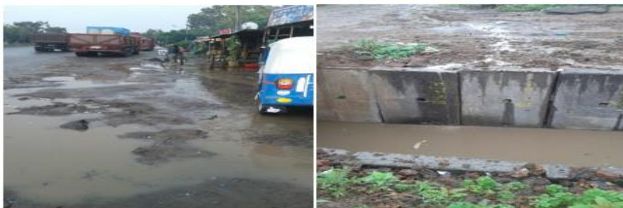
Figure 1-2 The drainage system problems on infrastructures
