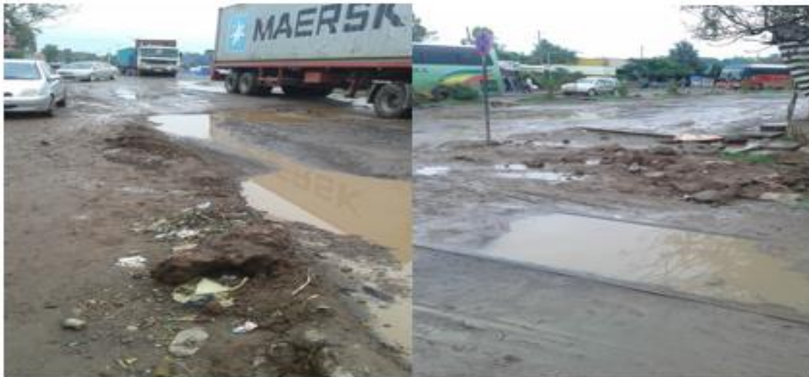
Figure 1-3 Silt loading and road failures by flood
