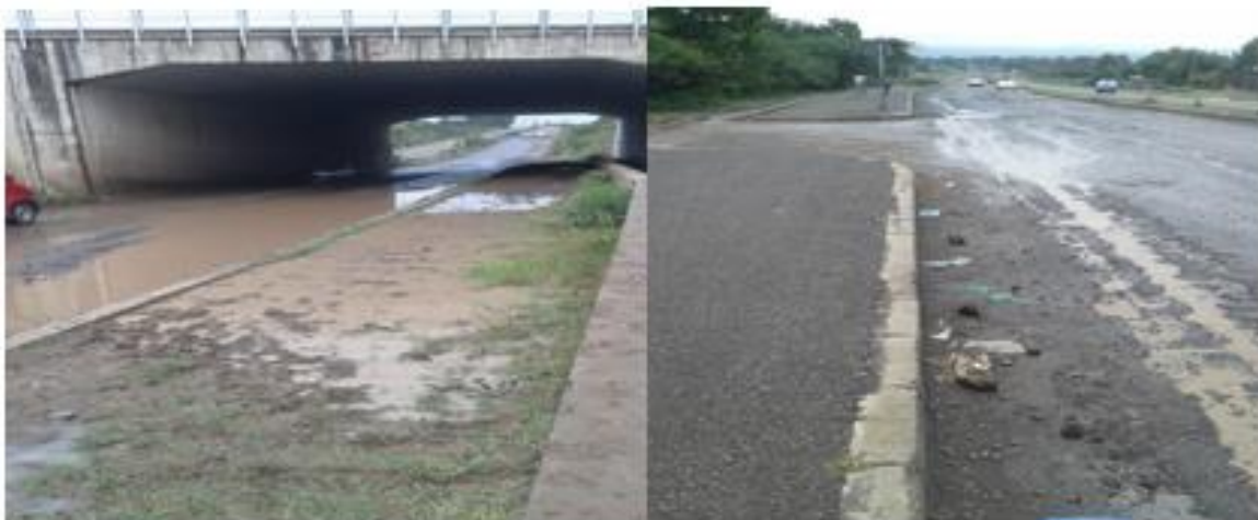
Figure 1-4 Water logging under bridge and flooding on the highway
