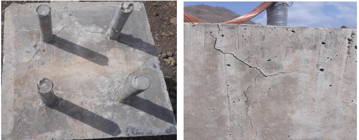
Figure1. 2 Equipment support foundation (0.8 m thick) cracking at top exposed surface and side surface.
