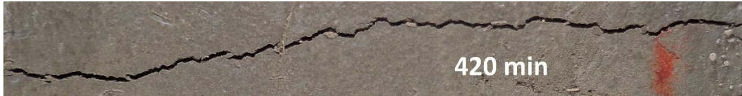
Figure 4-7 The propagated crack width of 0.035%
