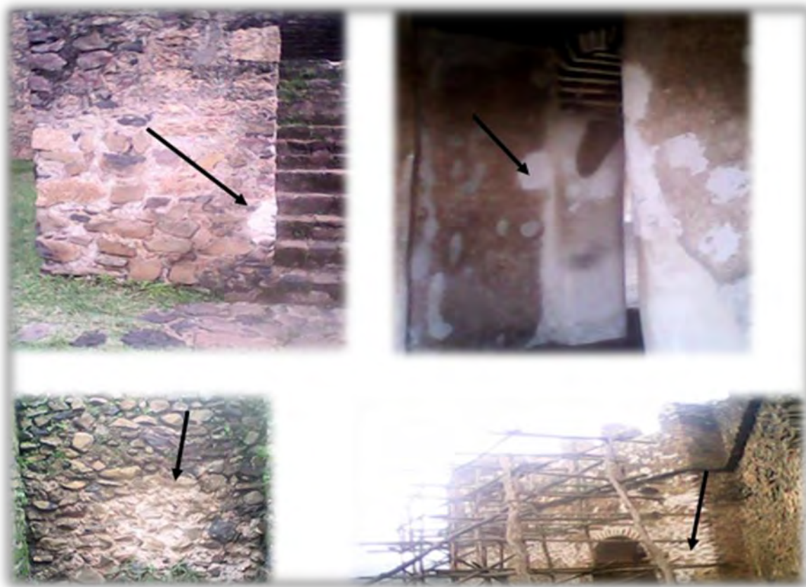
Figure 29: Mortar re-pointing in the internal and external appearance of the palace wall
