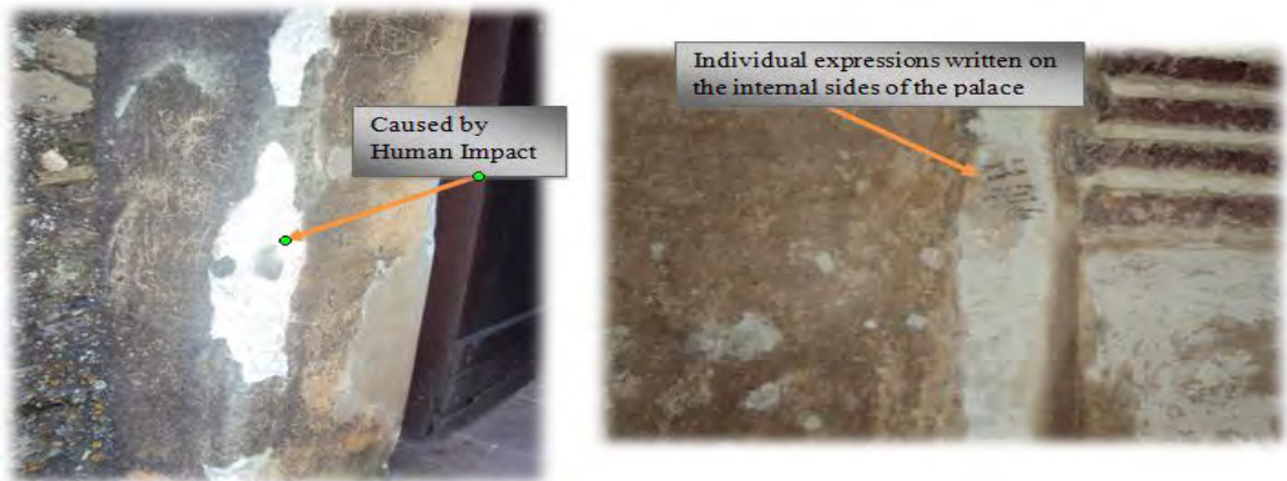
Figure 24: Mortar deterioration due to Mechanical action
