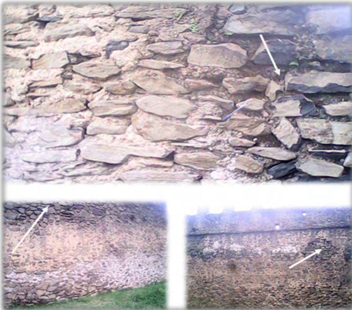
Figure 27: Some spotted sites which shows critical mortar deterioration
