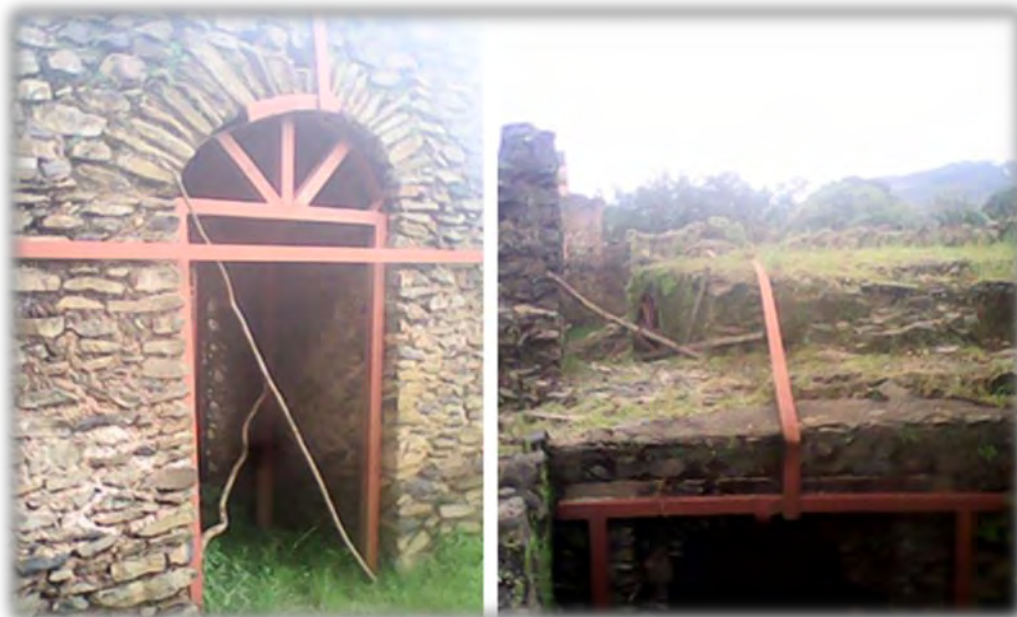
Figure 28 : Bracing steel in some specific wall portion
