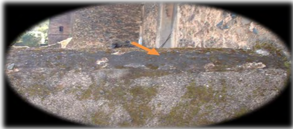
Figure 22: Mortar deterioration due to Chemical Reaction
