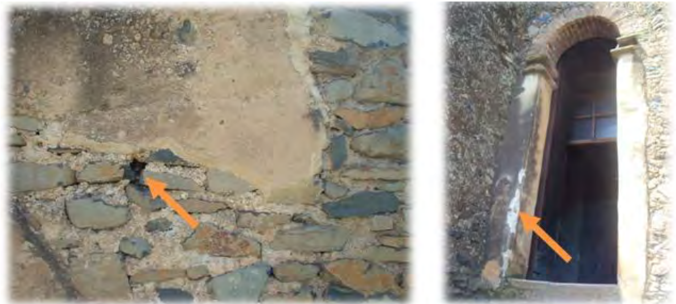
Figure 21: Deterioration of rendering Mortar
