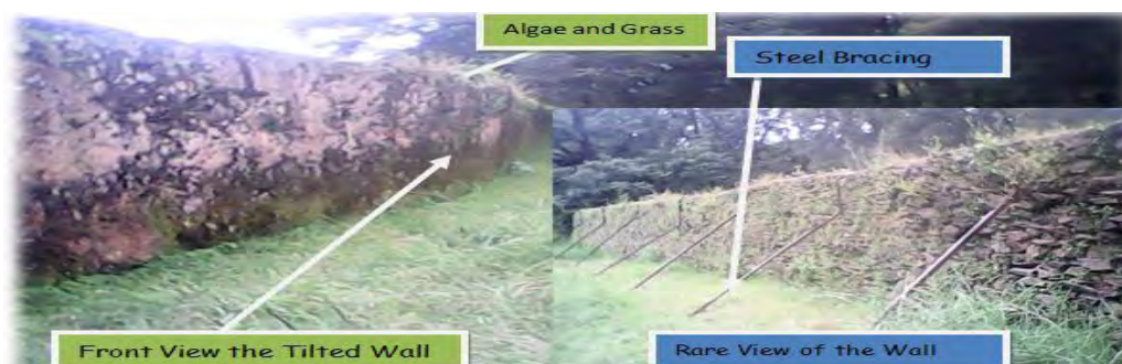
Figure 26: Leaning Of the Masonry Wall in the Royal Palace Near to the Main Road
