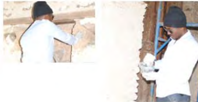
Figure 14: Sample taken from the internal wall
