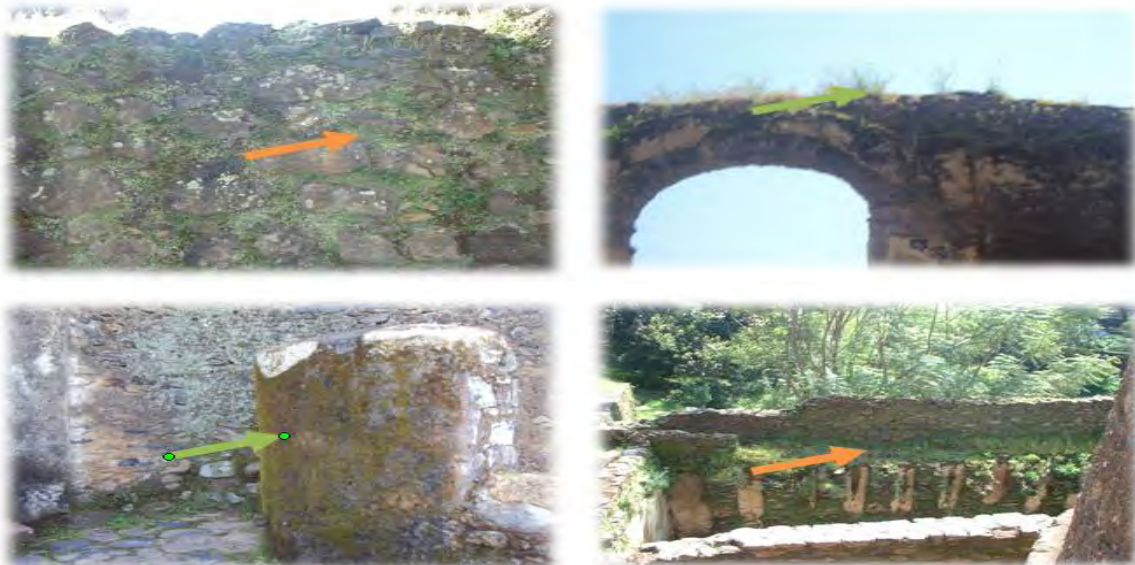
Figure 23: Mortar deterioration due to Biological Causes
