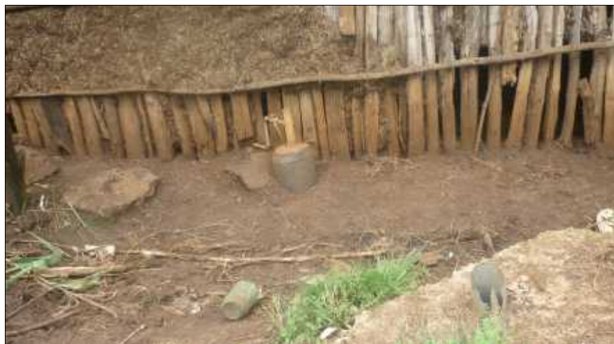
Figure 14b. Examples of improperly built toilet seats
