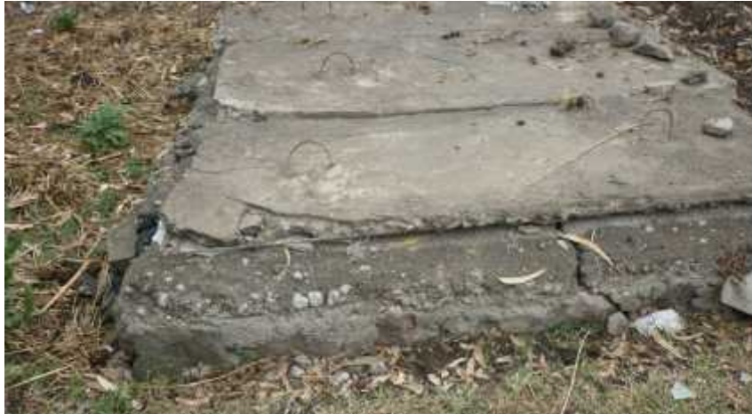
Figure 10. Cracking/fracturing of an outlet tank and slabs
