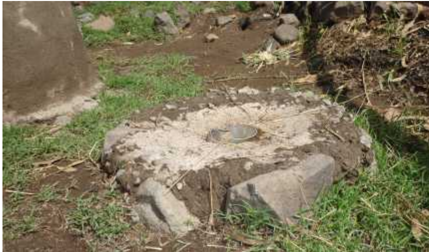
Figure 14a. Examples of improperly built toilet seats
