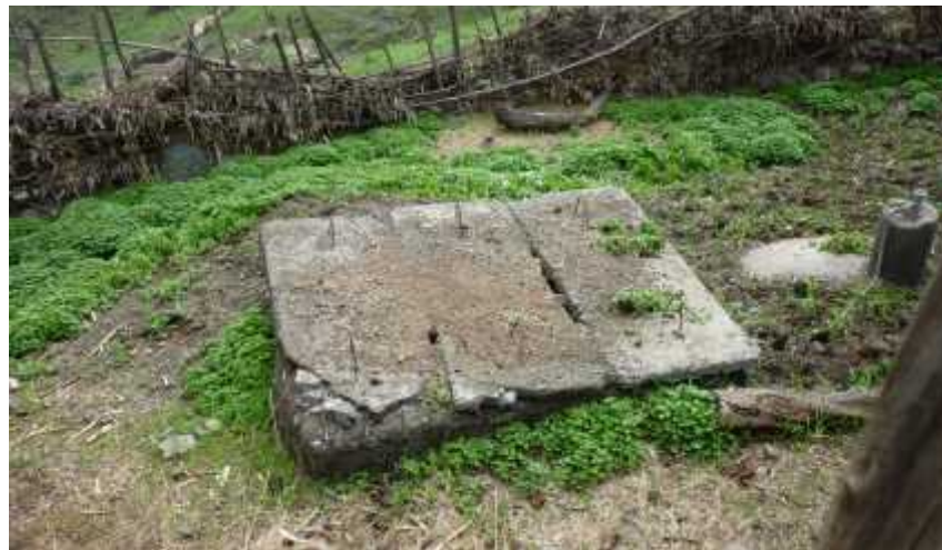
Figure 11. Fracturing of slabs
