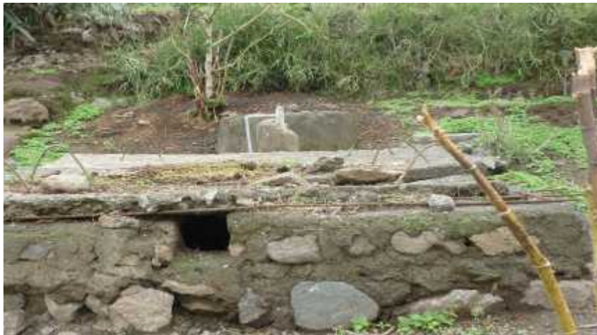
Figure 12. Improper biogas installation site selection
