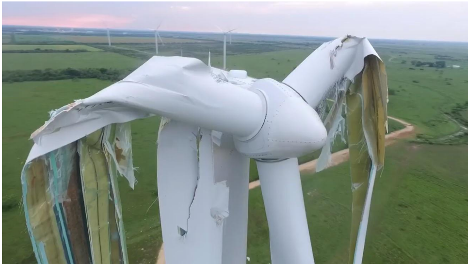
Figure 5: WTG destroyed in Texas as a result of high wind load (by Jeremy Rockit)
