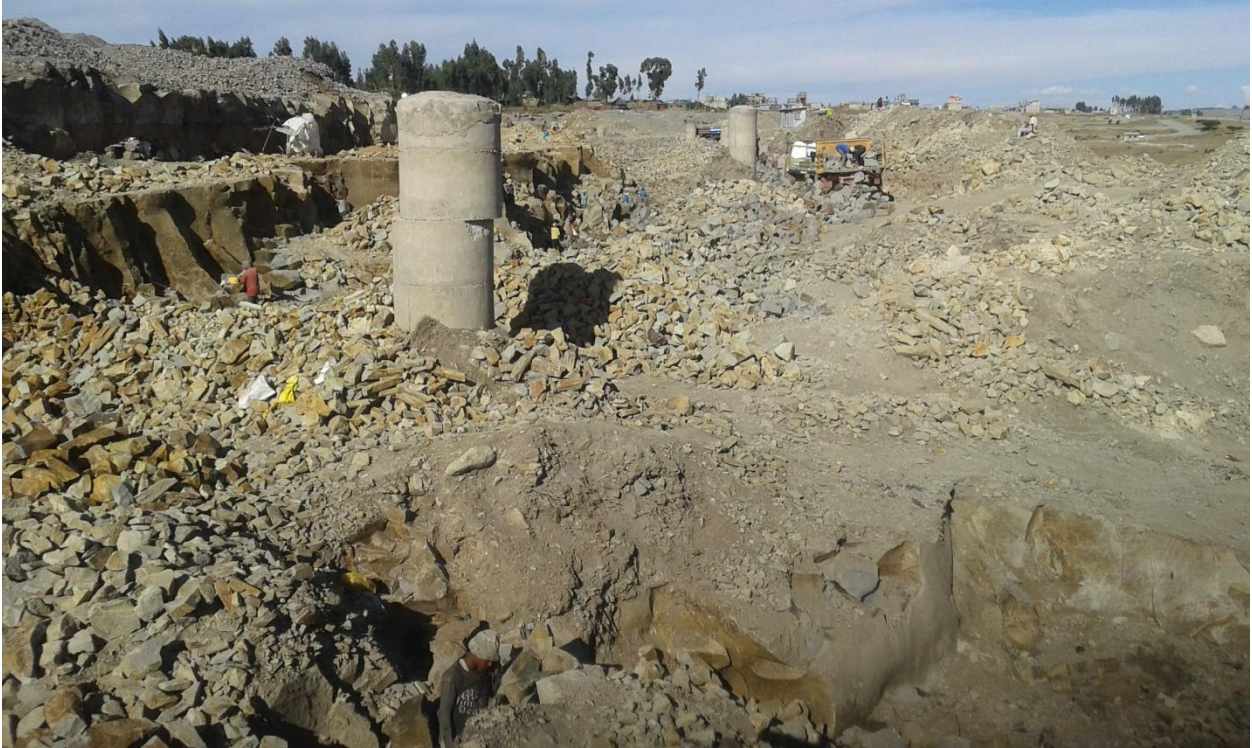
Plate 24 Constructed sewer line at Bole Qatla Quarry area exposed by quarrying
