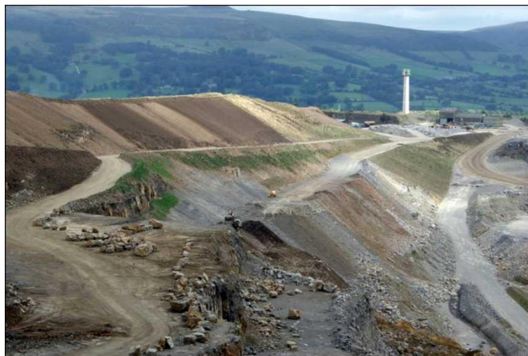
Plate4 An example of rollover slopes being formed at the Hope Cement Works, Hope, Derbyshire, England. The technique was used in a progressive reclamation scheme to cover a number of benches where extraction has ceased.
