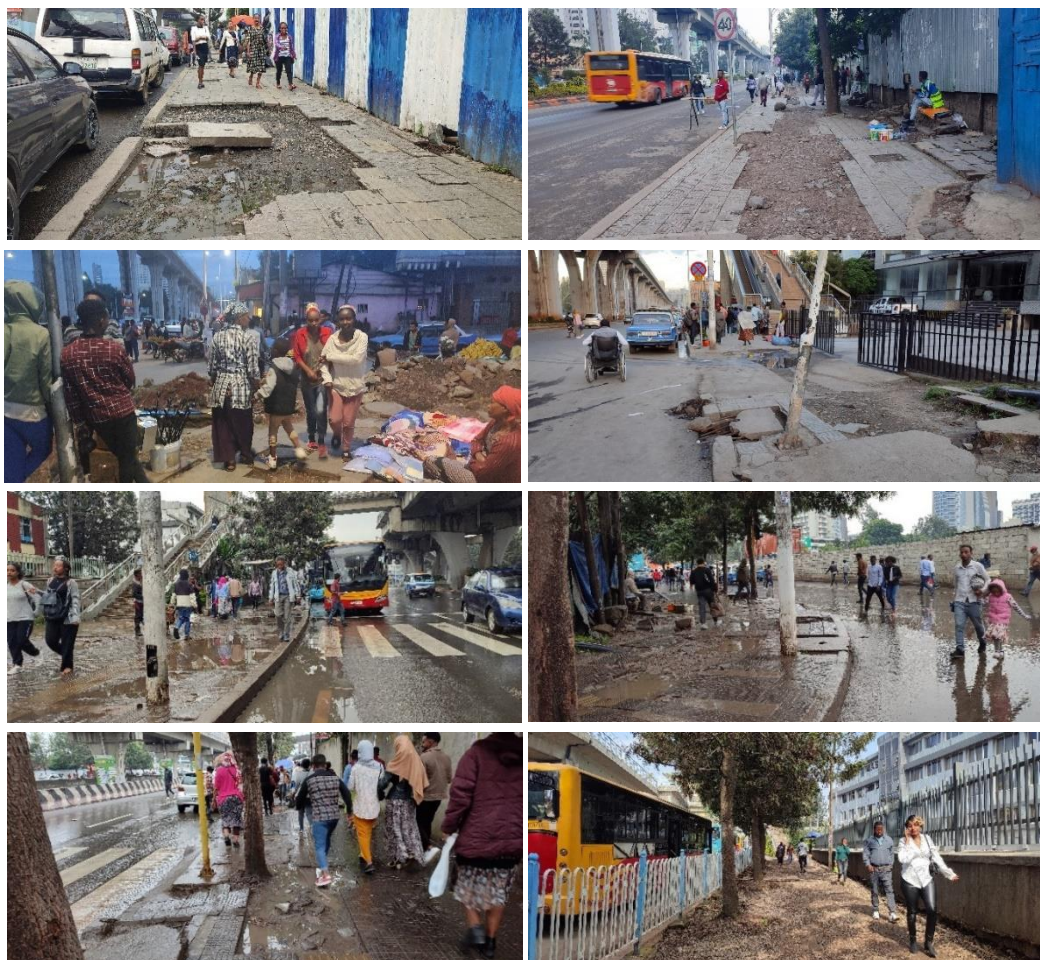
Figure 4.28 Unpaved and/or deteriorated pavement condition
