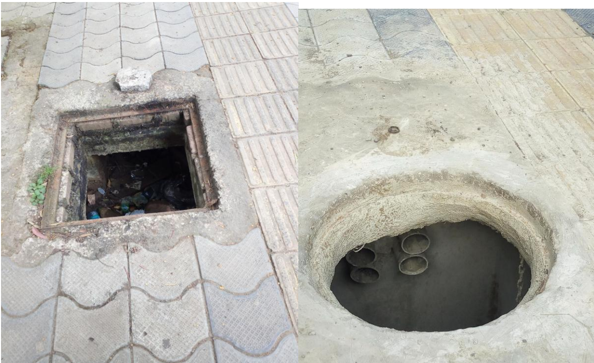
Figures showing potholes on the sidewalk
