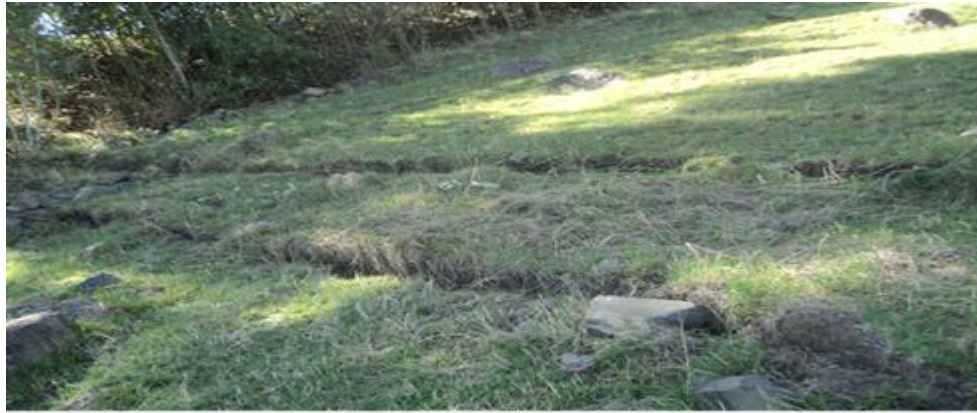
Figure 2.17 Tensional cracks down the road at Shola Wuha locality
