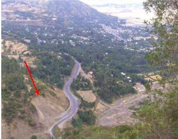
(a) Landslide which has fallen in steep slope cut (Wurgessa)
