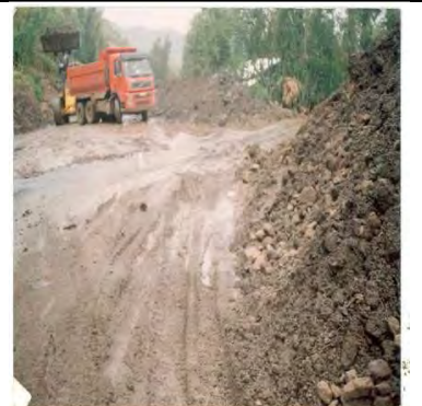
(k) The road affected by debris flow
