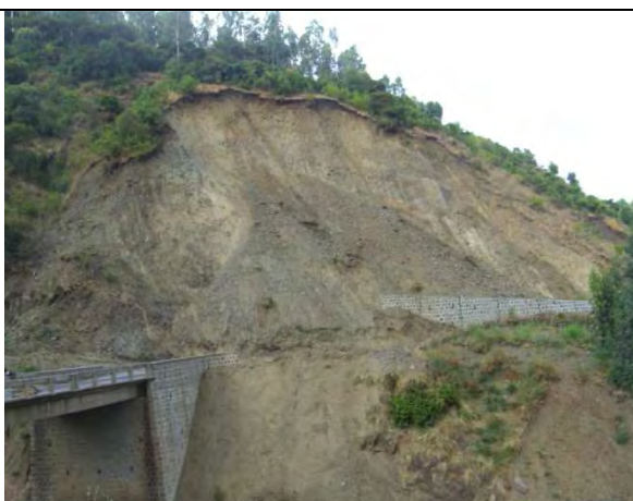
(e) Landslide which has affected retaining wall near Golo stream bridge (Wurgessa).
