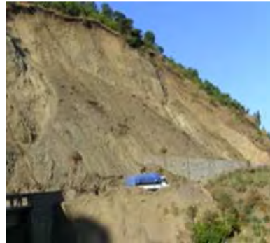
(e) Retaining wall affected by the landslide at the main bridge of Golo River (Wurgessa).
