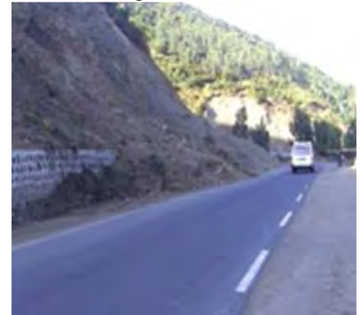
(f) Retaining wall affected by the landslide (Wurgessa).
