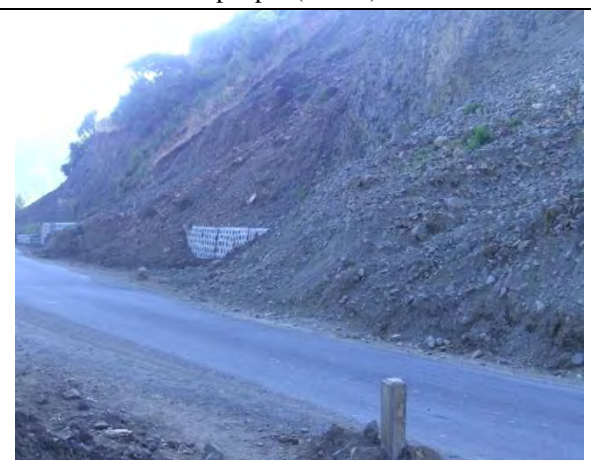
(f) Retaining wall affected by colluvial slide (Wurgessa near Golo stream).
