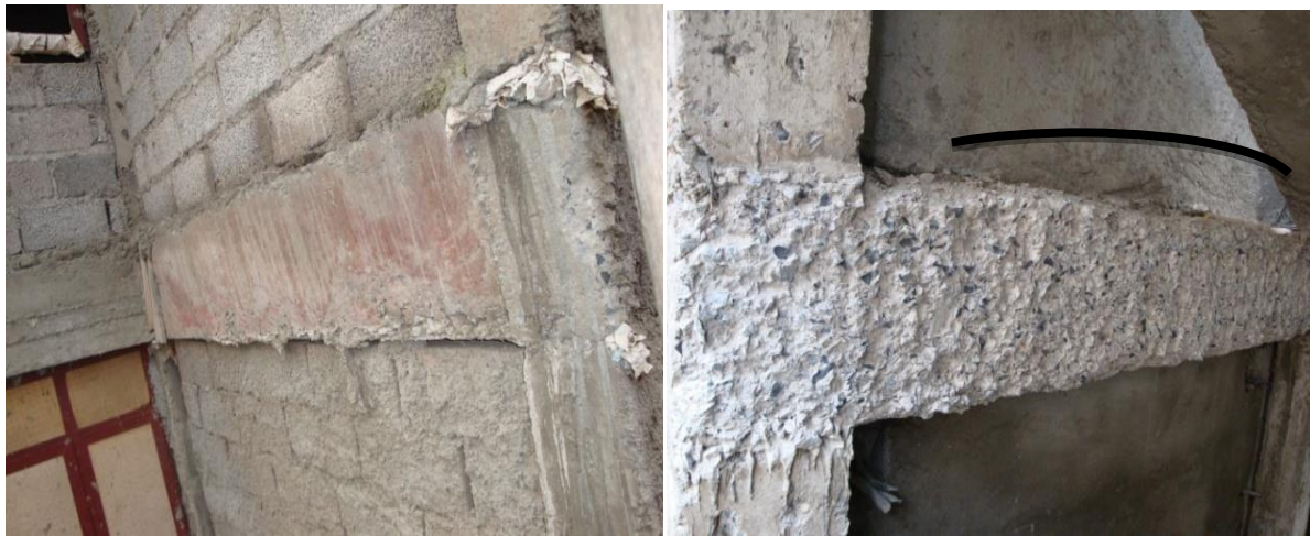
Misalignment between wall and beam Bended beam because of improper form working
