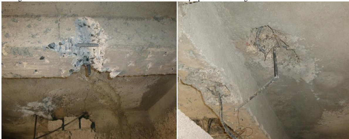
Figure 2. 3 Construction of structural quality problems and defects (Addis Ababa)
