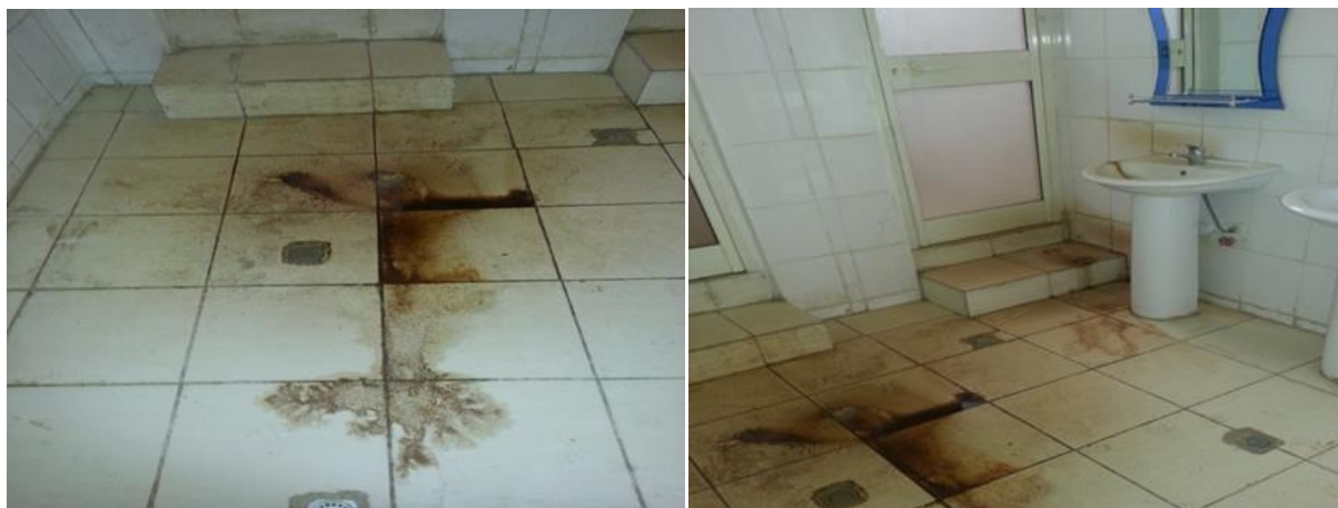
Figure 2. 5 Finishing work and sanitary pipe lines failure happened immediately after completion of the work (Addis Ababa)
