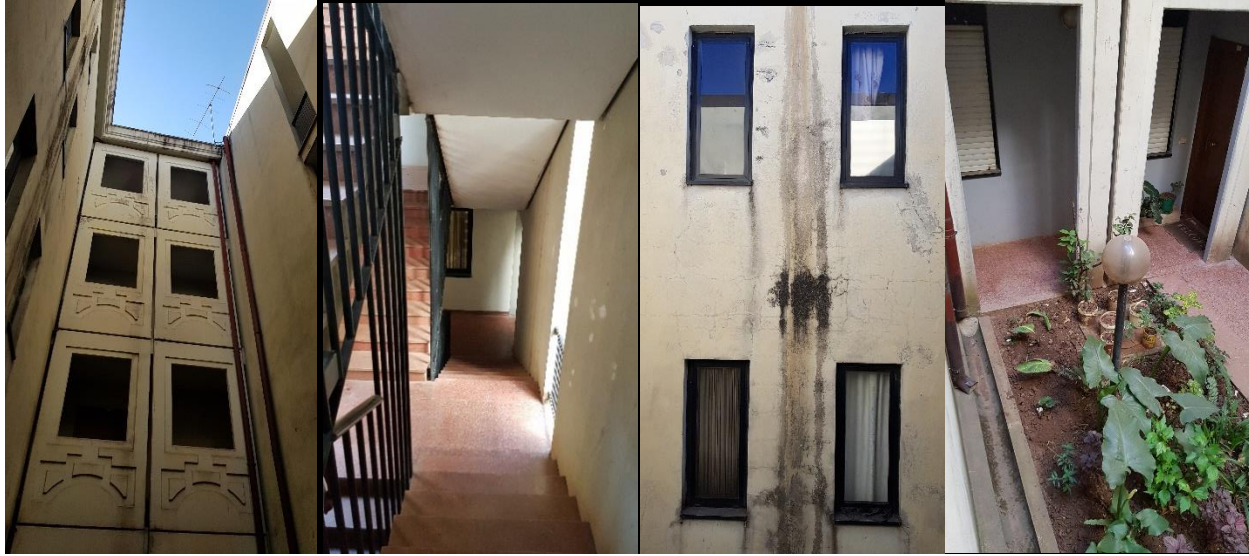
Figure 40: Open down, naturally ventilated and lighted staircase, Dampness and microbial growth and green area in the ground floor of the open down (from left to right)
