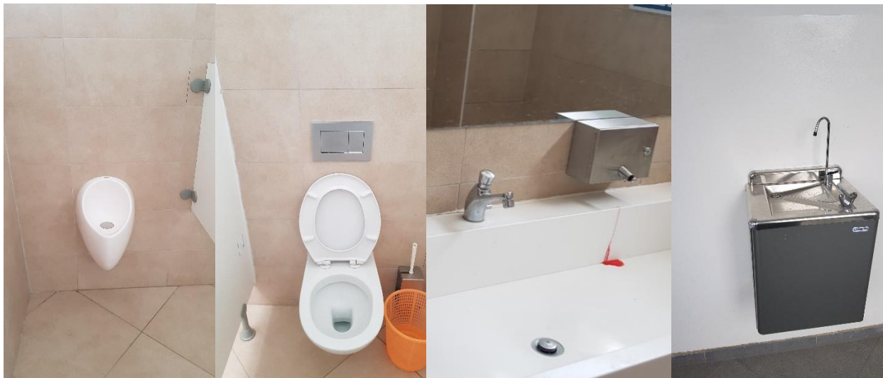
Figure 18: waterless urinals, dual flushing, and auto-shutoff sinks (left to right)
