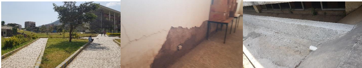
Figure 28: Pavement around the building (left), the effect of the recurring flooding in the basement (middle) and prevention method for the flooding (right)
