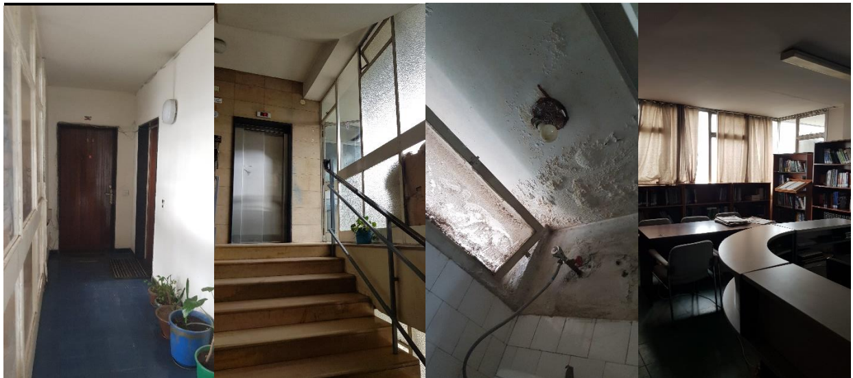
Figure 54: Naturally lighted circulation, Dampness in the toilets, closed curtain on the front side due to harsh sun (left to right)
