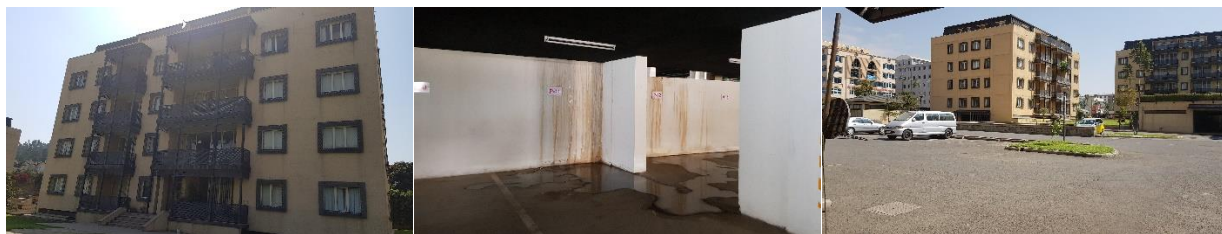
Figure 36: The front side of the building studied (left), Water leakage in the parking garage with green roof (middle) and Part of the compound (right)
