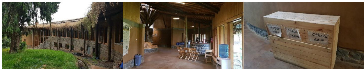
Figure 13: Exterior materials (left), Interior materials (middle) and Waste disposal bin (right)
