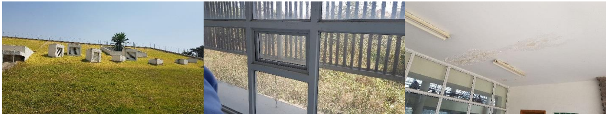
Figure 32: Opening for ventilation and lighting (left), Limited operable windows (middle) and water leakage from the green roof (right)
