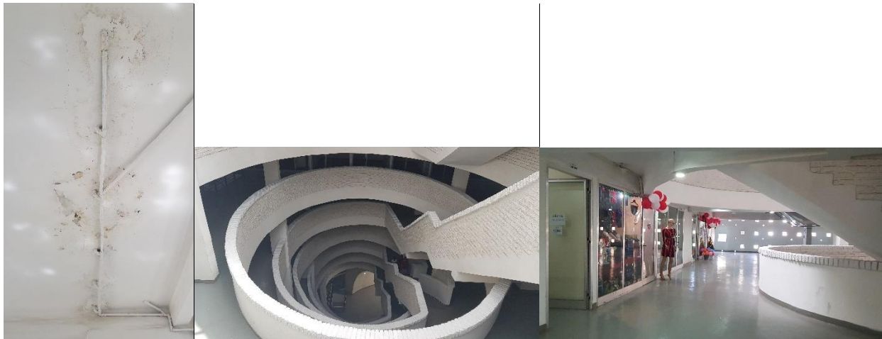
Figure 26: Dampness problem (left), open down to the main entrance (middle) and shops inside the building (right)
