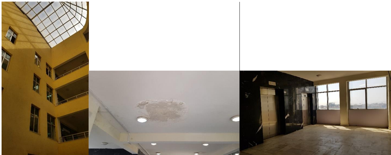
Figure 44: Open down all the way to the ground floor with skylight (left), Dampness in the building (middle) and well-lighted circulation (right)
