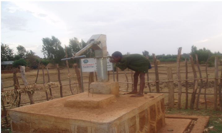
Fig 6.4 Non-functional well, Zekuskuam, near Wetet Abay (Gps location 288515mN, 1258795mE)
