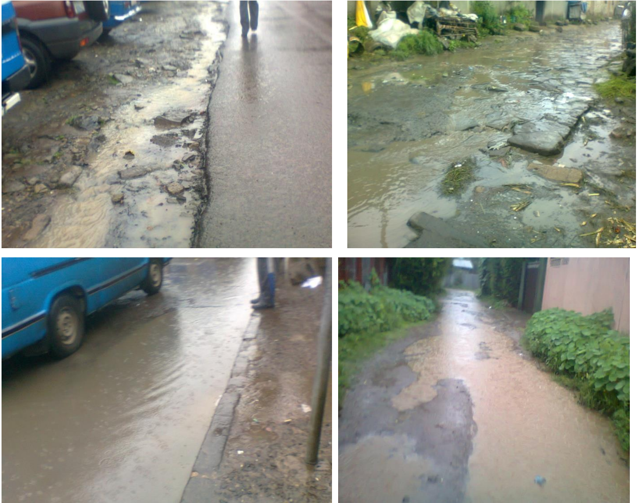
Figure 4.7 Flood over major and minor streets of the three woredas (source field survey, 2012)
