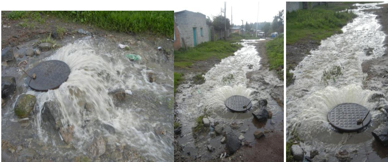
Figure 4.16 Flow over manholes in woreda 7 (source: Field survey July, 2012).
