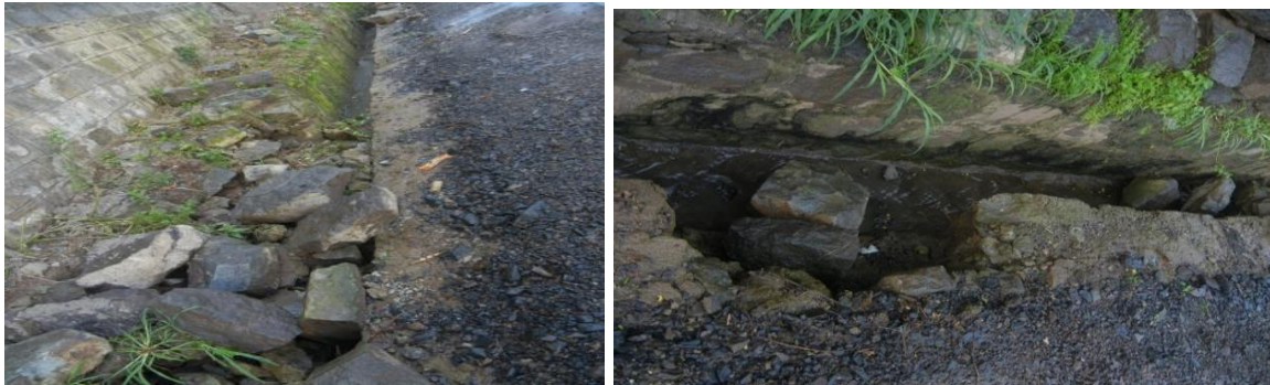
Figure 4.15 Failed drainage ditches in woreda 6 (source: Field survey July, 2012).
