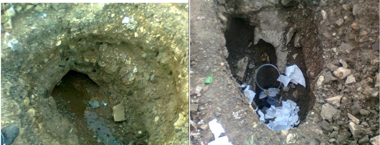
Figure 4.17 Blocked drainage networks in woreda 6 and 8(source: Field survey July, 2012).
