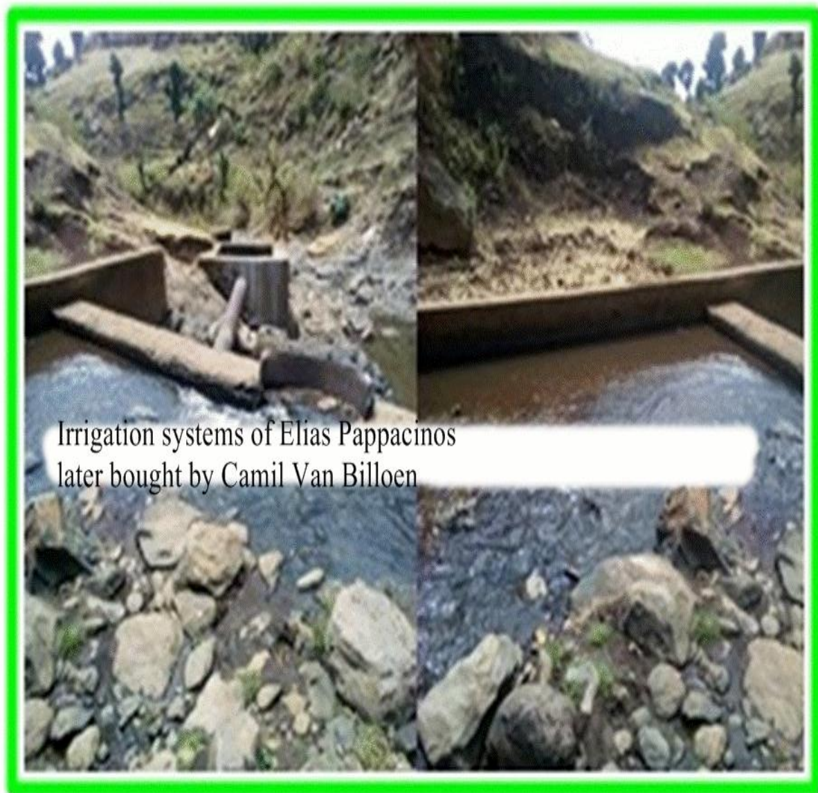
Figure 3.5: On-site water storages, water inlets to storages and irrigation channels
