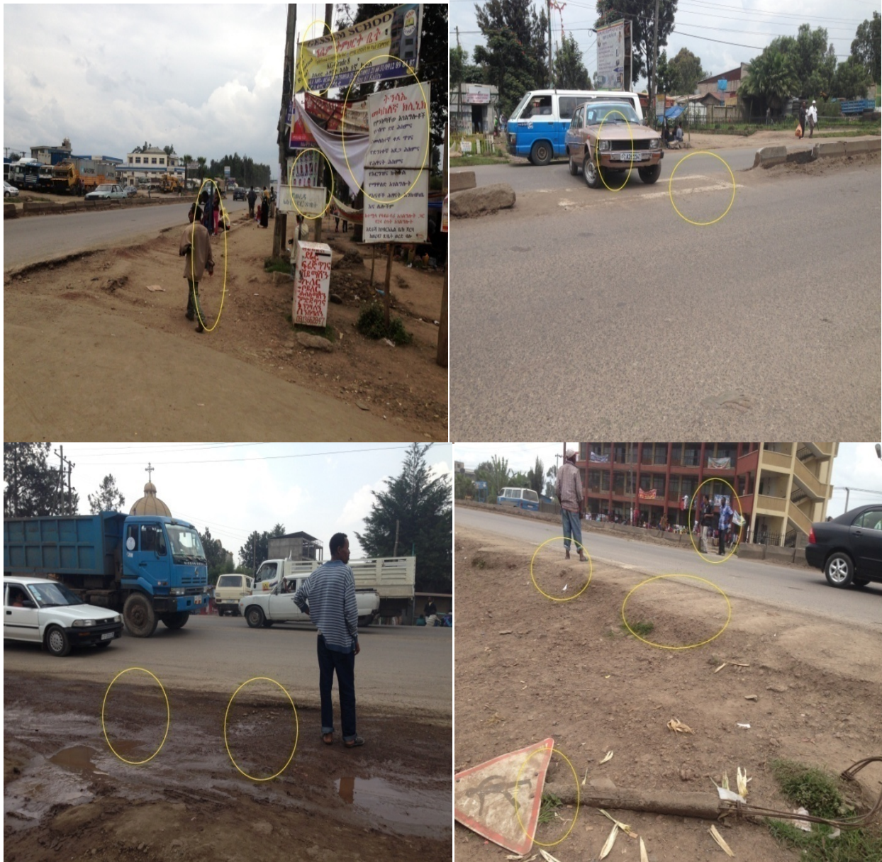
Figure 47. Photo. Pond of water at the Carriageway, Shoulder and pedestrian walkway missing, complete absence of lane marking (edge line, median, transverse markings), there were completely absence of pedestrian crossing warning a head sign, and lack of maintenance.
