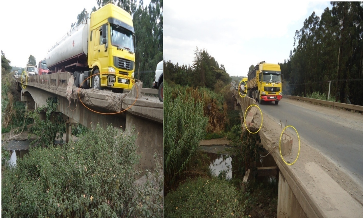
Figure 37.Photo. Bridge damage by vehicles' (collision with roadside objects), lack of maintenance, and create high potential safety problems to vehicle drivers and vulnerable road users
