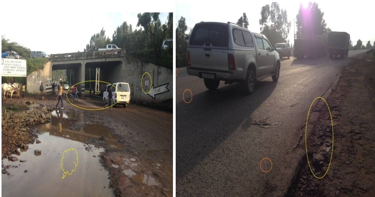
Figure 35.Photo. Poor drainage systems, pond of water at the Carriageway pedestrians trying to deal with the water obstacle fail to observe approaching vehicles, complete absence of lane markings (edge line, median, transverse markings) and vehicle height limit Warning sign not located at appropriate location ,beside this the sign is also worn out.
