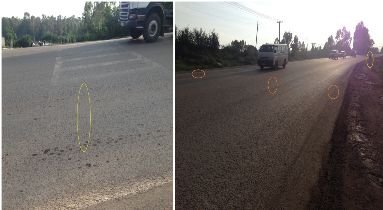
Figure 34.Photo. Faded and invisible pedestrian crossing markings, complete absence of lane marking (edge line, median markings, transverse), and no pedestrian walkway
