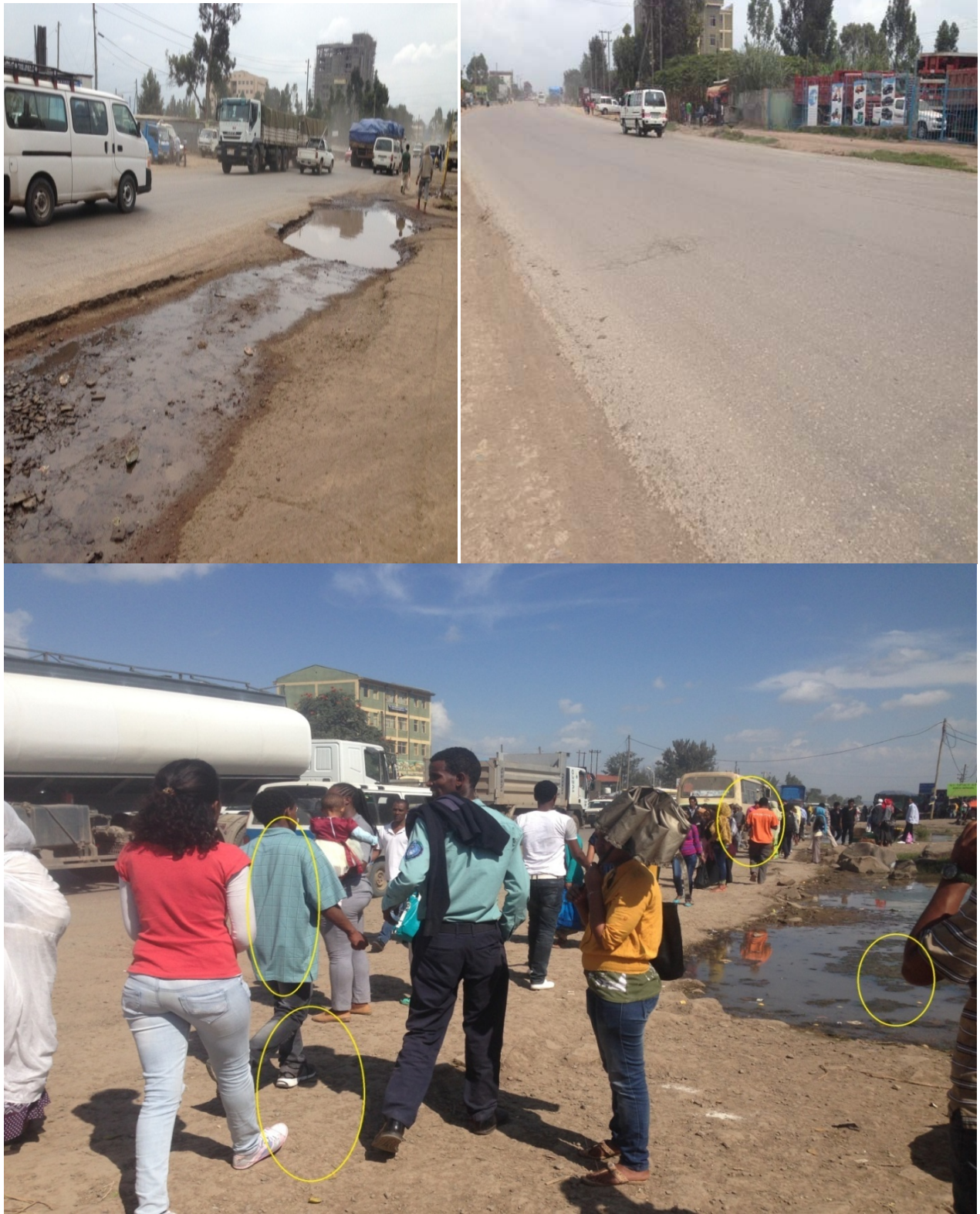
Figure 39.Photo. Pond of water at the Shoulder and pedestrian walkway, complete absence of lane marking (edge line, median, transverse markings); there were completely absence of pedestrian crossing warning a head sign, and lack of maintenance.
