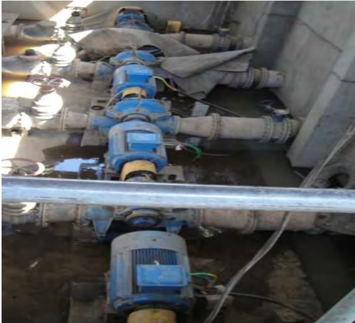
Figure 4.2 Installed pumps at Fentale-Qawa Pump Station
