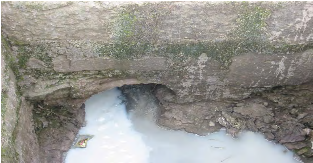
Figure3.3: Waste water collection site.
