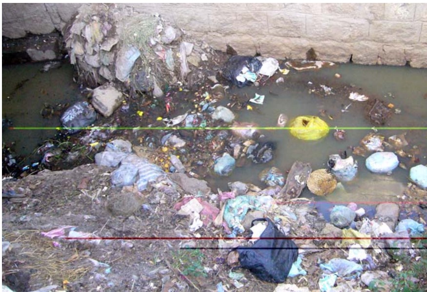
Figure 4.10: An Open Ditch Filled with Sewer and Plastic Bags, Possibly with Human Waste. (Tureta Sefer: 2007)
