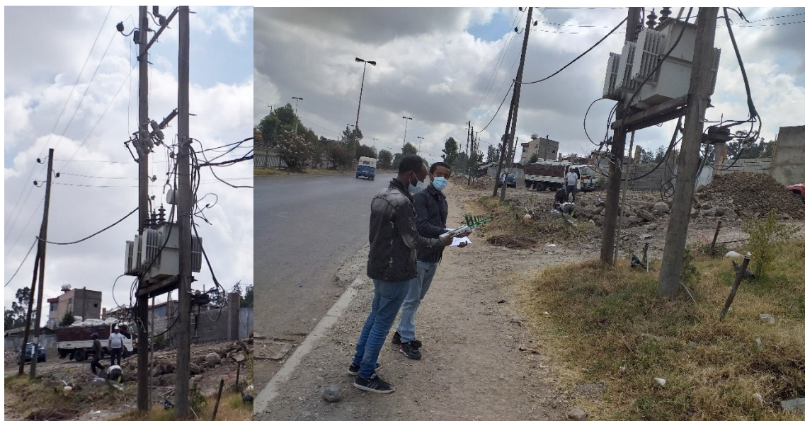
Figure 26: 100kv transformer around Haile garment round about
