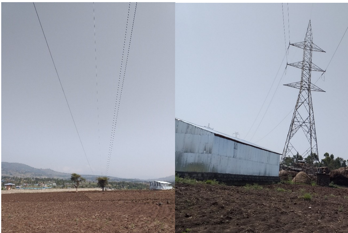
Figure 21: 132kv HVPL around Gelan area
