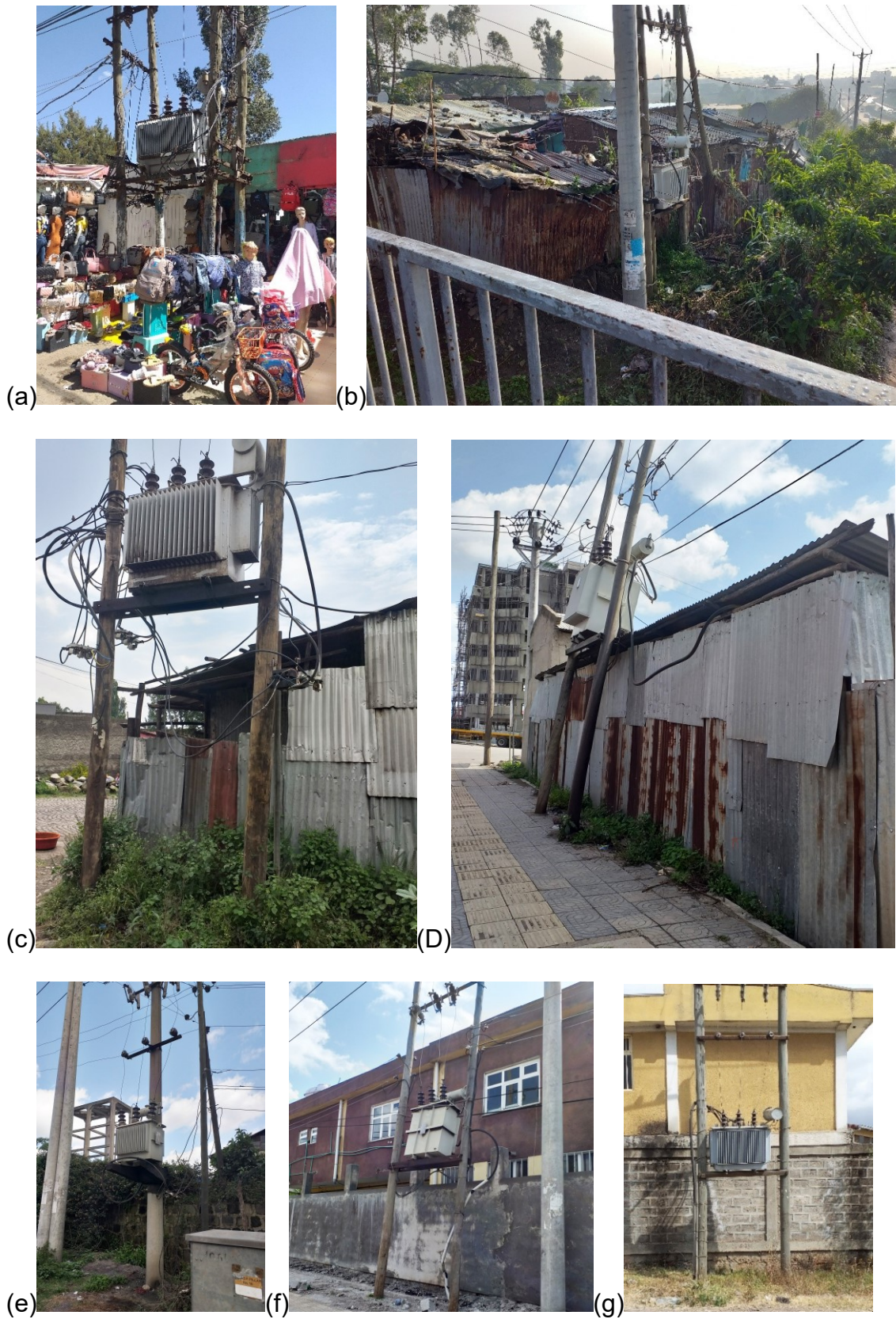
Figure 12: (a)-(g) Transformer and building relation in Addis Ababa at different places (a) around 22, (b) Hana Dildiy, (c) Dufa Dufa, (d) & (f) Kadisco, (e) Maseitegna, & (g) Haile Garment.
