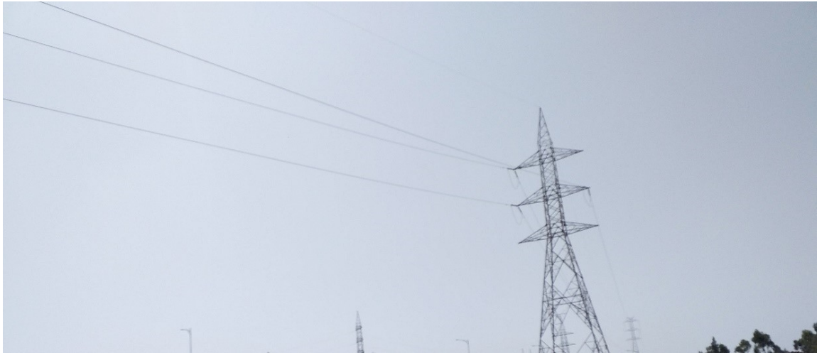
Figure 19: 230Kv high voltage powerline
