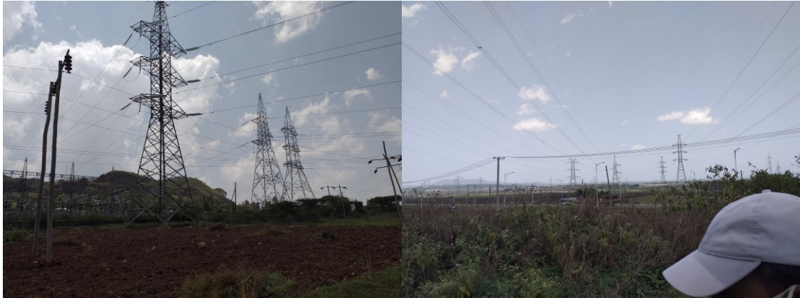
Figure 9: High power transmission lines in Kality I substation
