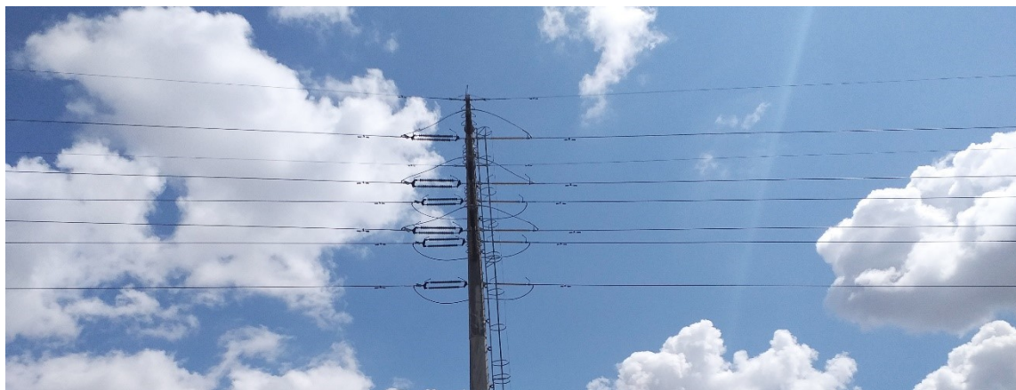
Figure 23: 45kv transmission line around Gelan area
