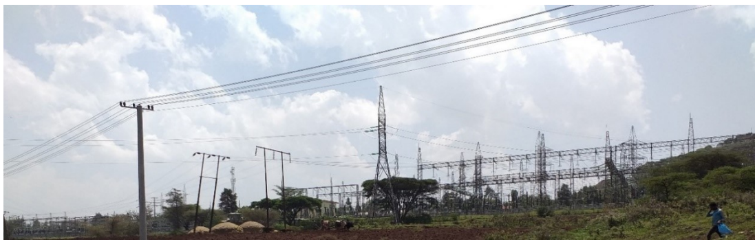
Figure 35: Akaki I substation side view
