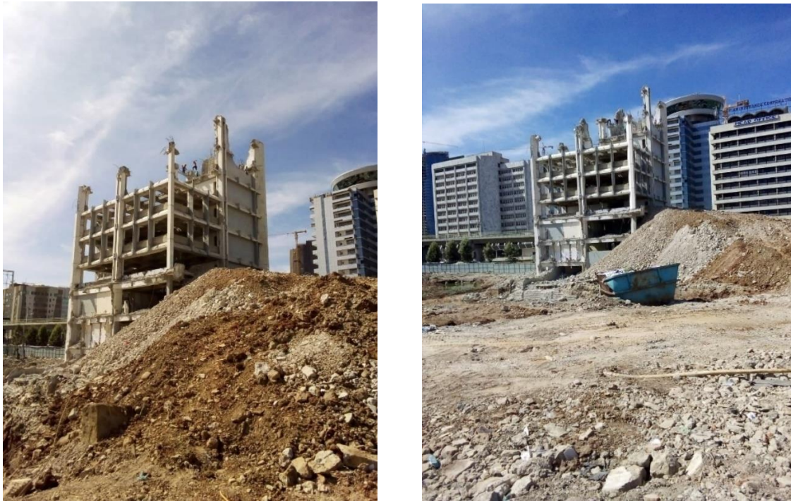
Fig. 4.10 (b) Demolition of Ethiopian Shipping & Logistics Services Enterprise building, Feb., 2020 (Source: self-taken)
