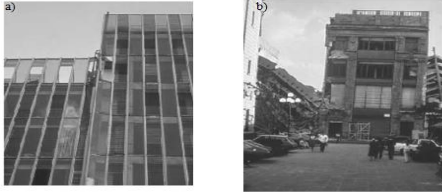
Figure 12: Damage of adjacent building due to pounding (Mexico 1985) [14]
