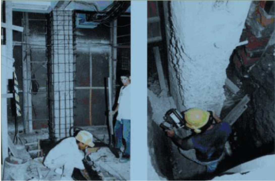
Figure 44 Installation of reinforced concrete jackets from the foundation level up to the beam soffit; examples from Colombia (source: WHE-2006-03, 2006).
