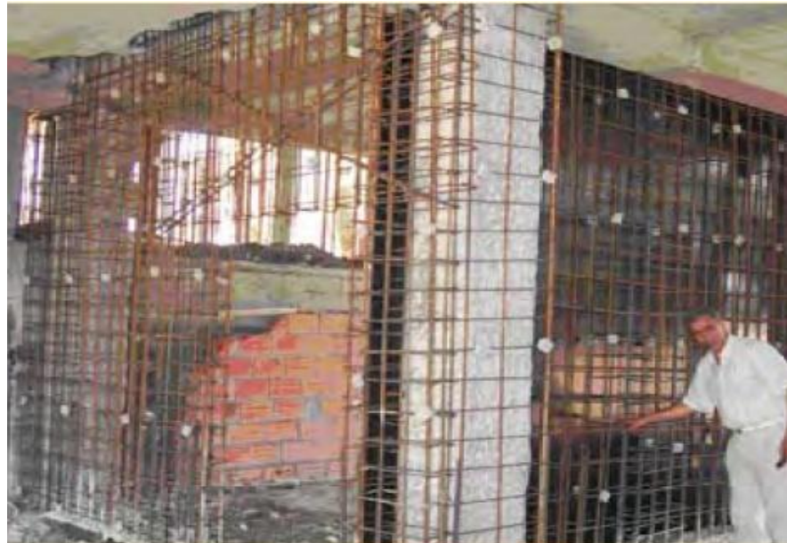
Figure 40 Retrofit of existing RC building using new RC shear walls and jacketing of the existing columns after the 2003 Boumerdes (Algeria) earthquake (photo: M. Farsi; drawing courtesy of CTC Algiers). Addition of new structural elements.
