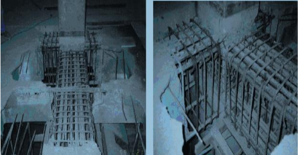
Figure 45 Jacketing of a beam-column joint region; an example from Colombia (source: WHE-2006-03, 2006).
