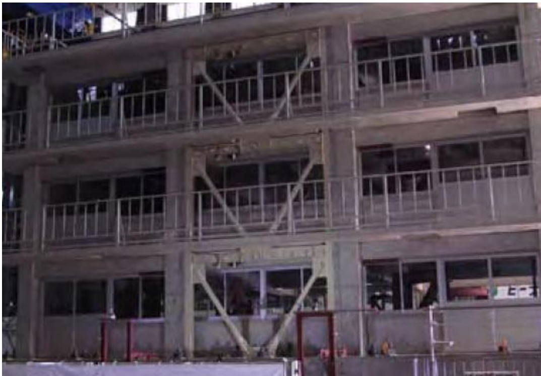
Figure 42 Retrofit of RC frames with steel braces – shake-table testing at E-Defence, Japan:
