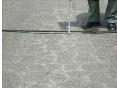
b) Ruts associated with cracks
