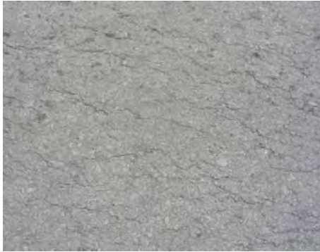
a) Dry and Brittle Surface
