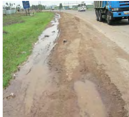
d) Side Drain Problem
