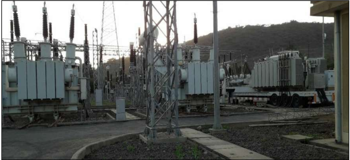
Figure 3-2 Existing Adama 2 and Mobile Substation
