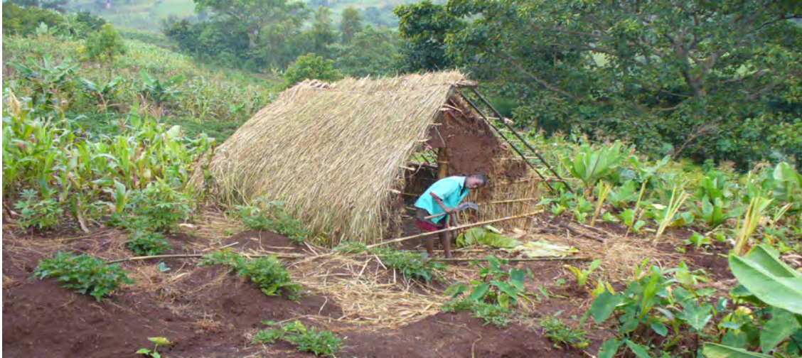
Fig. 10 Basketo youngster constructing a hut on the lower portion of his father's garden. Note that the recently planted enset is at the lower side. Such rectangular house is temporary and eventually to be replaced by a circular one (Photo: Feleke Woldeyes)
