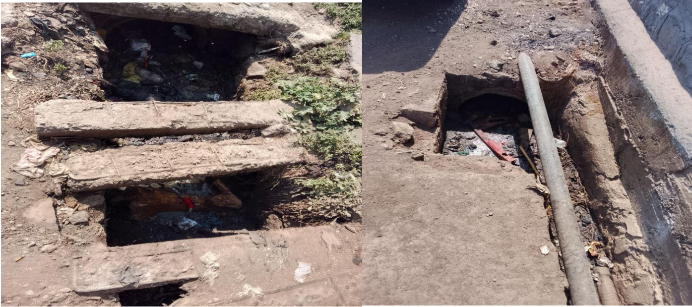
Figure 1-3: The image on the right and left show solid waste accumulation in open drainage system
