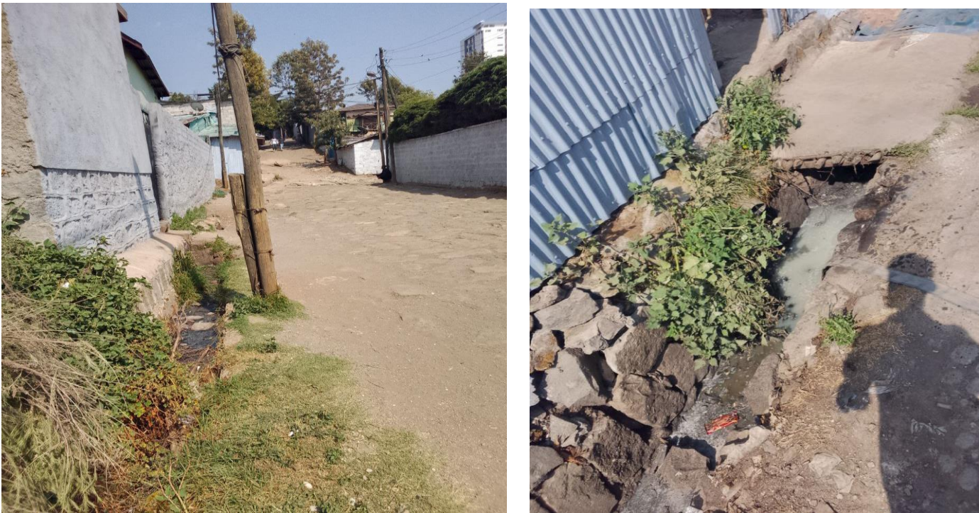
Figure 1-2: improper conveyance of open drainage flow in the left and right images
