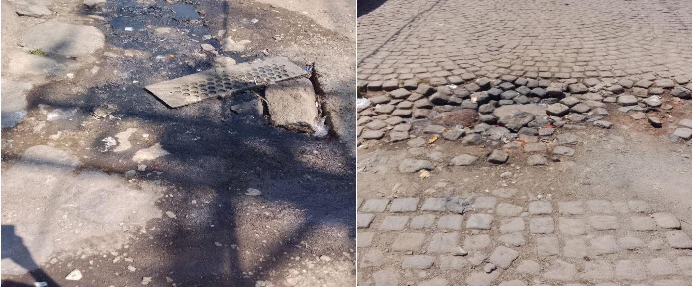
Figure1-1: The images on the right and left show that the drainage system is surcharged and, and flowing over the surface
