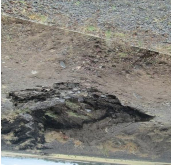
Figure.4.2 Lack of drainage facility
