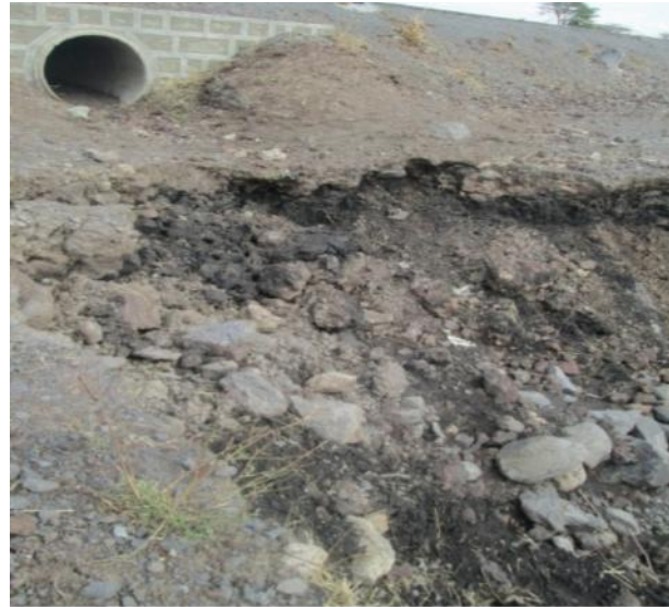
Figure 4.3 Improper drainage facility
