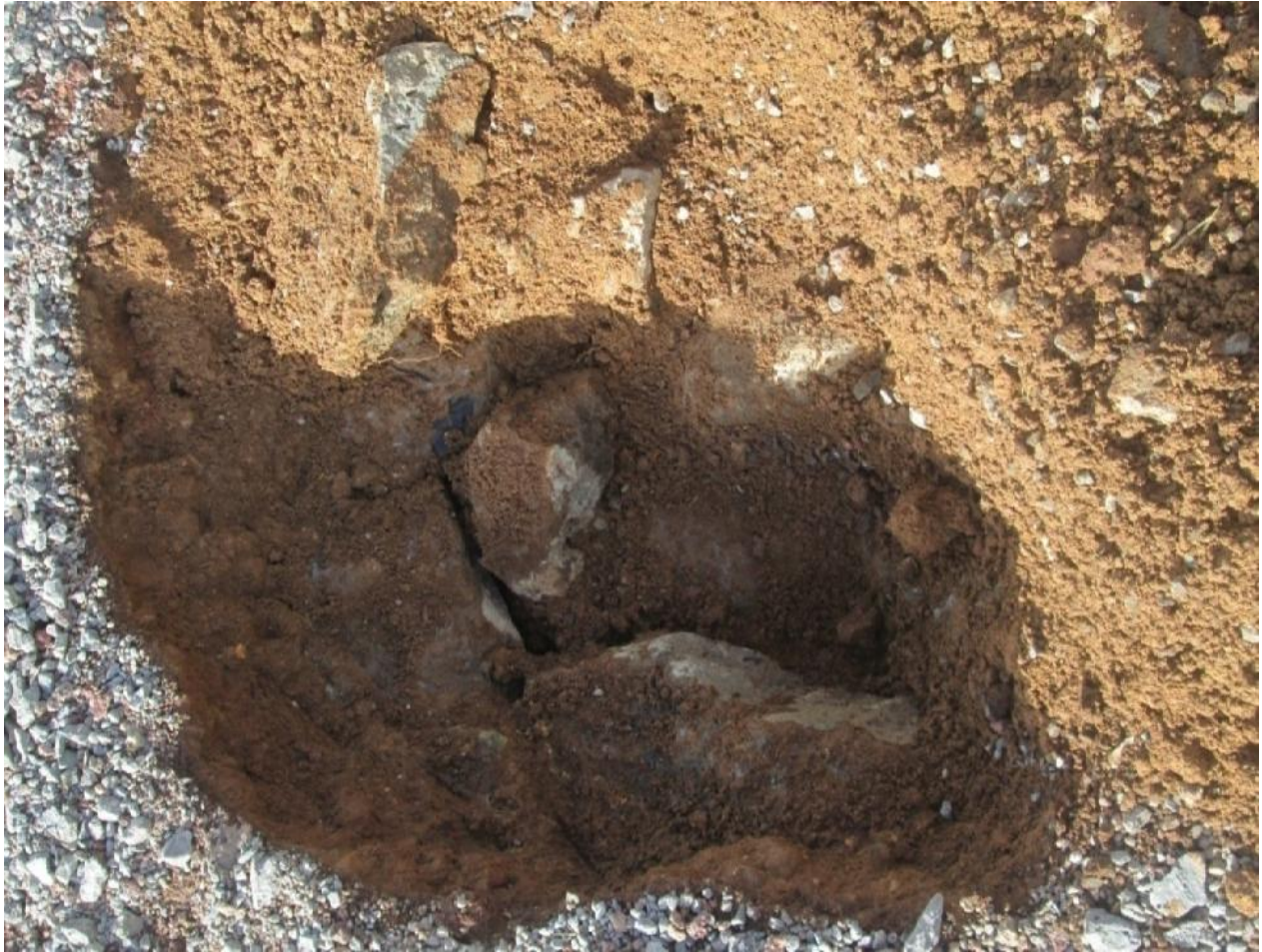
Figure 4.1 Exposed fill materials where the rock floats on the fine materials below embankment around station 24+560
