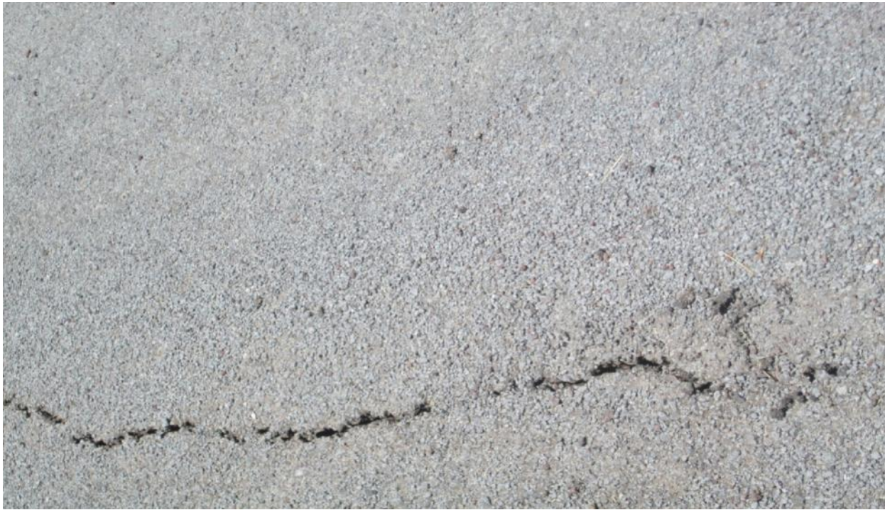
Photo 4 Surface cracks at station 10 + 346 – 10 + 600 LHS
