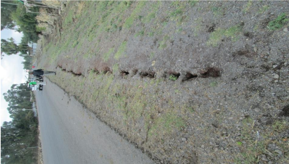
Photo 2 Edge cracks at station 28 + 600 RHS
