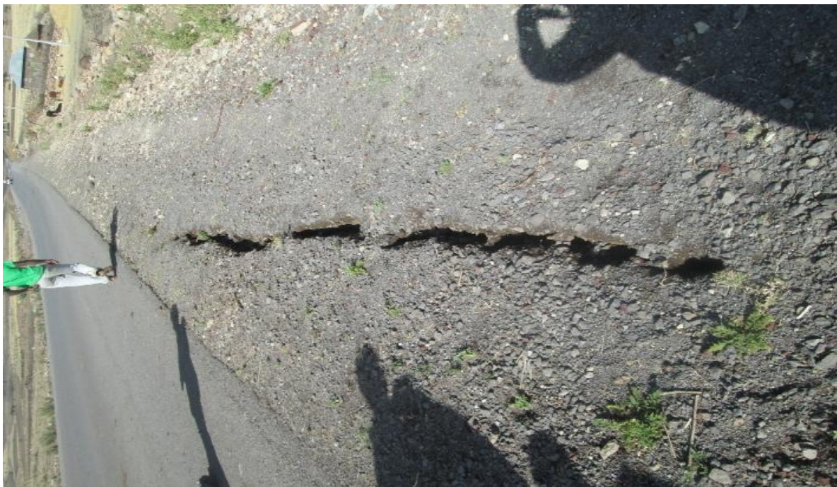
Photo 3 Edge cracks at station 24 + 590 – 24 + 610 RHS
