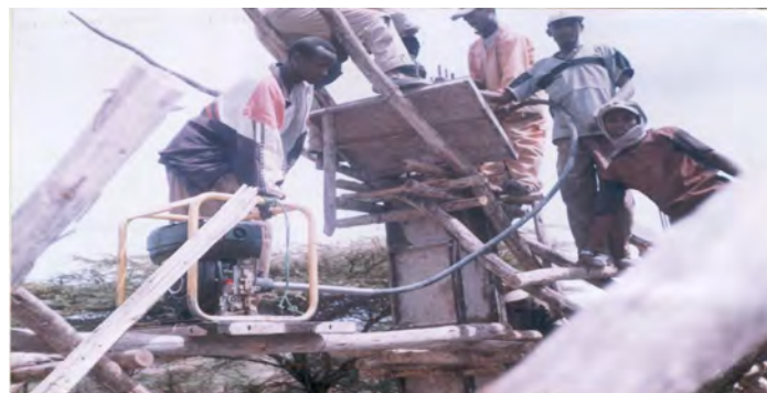
Fig 4.6 Compaction of concrete on ground column of Nazareth Technical college building project
