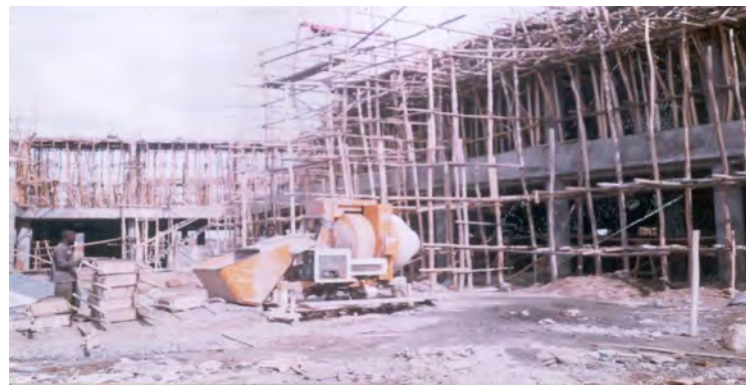
Fig 4.5 300liters stationary concrete mixer used on the building project of Oromyia Regional State President Office, Adama
