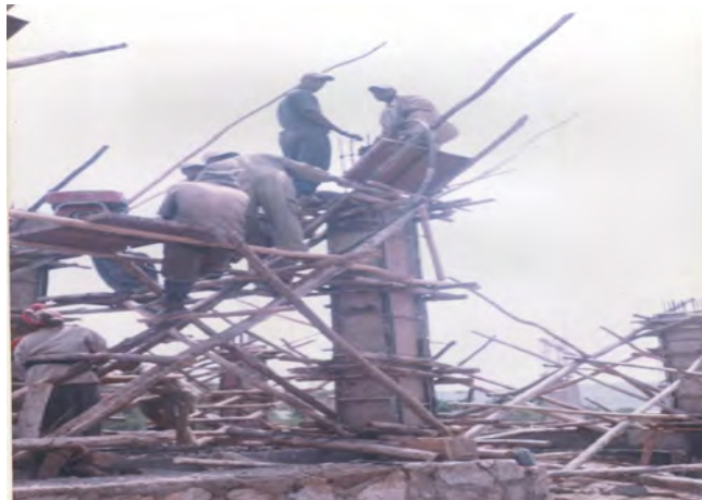
Fig 4.7 concrete placing & compaction on ground column of Nazareth Technical college building project
