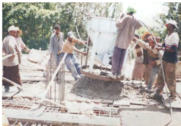
Fig 4.9 Placing of concrete on the slab of the building project of Addis Ababa University, Faculty of Veterinary medicine, Debrezeit.
