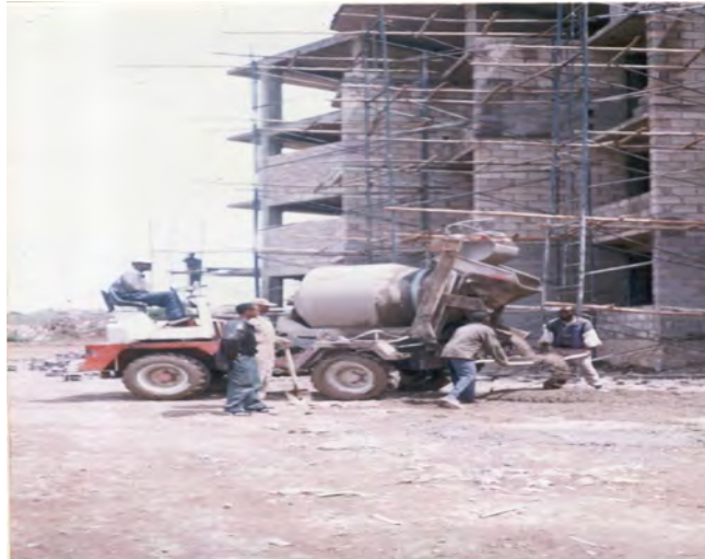
Fig 4.8 Concrete mixing & discharging operation with a self loading tractor on Nazareth Technical college building project
