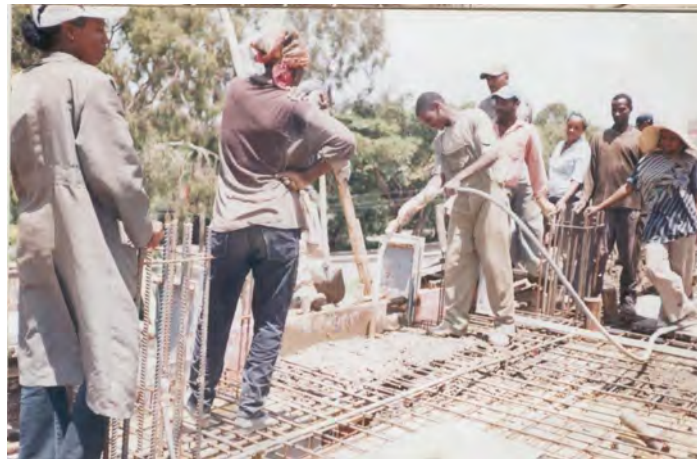
Fig 4.10 Compaction of second floor slab concrete on the building project of Addis Ababa University, Faculty of Veterinary medicine, Debrezeit.
