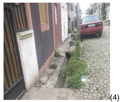
Fig4.11a (1) Untreated open space (2) Frontage garden (3) Inactive road (4) Open Concrete ditch.
