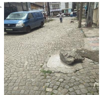
Fig 4.2b Typical 8m Coble stone road with sewerage line
