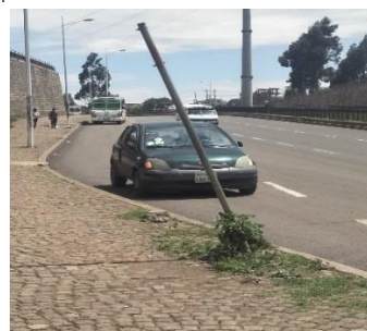
Fig 4.2d Typical 40m asphalt road with side walkway paved with Coble stone and greenery at the median
