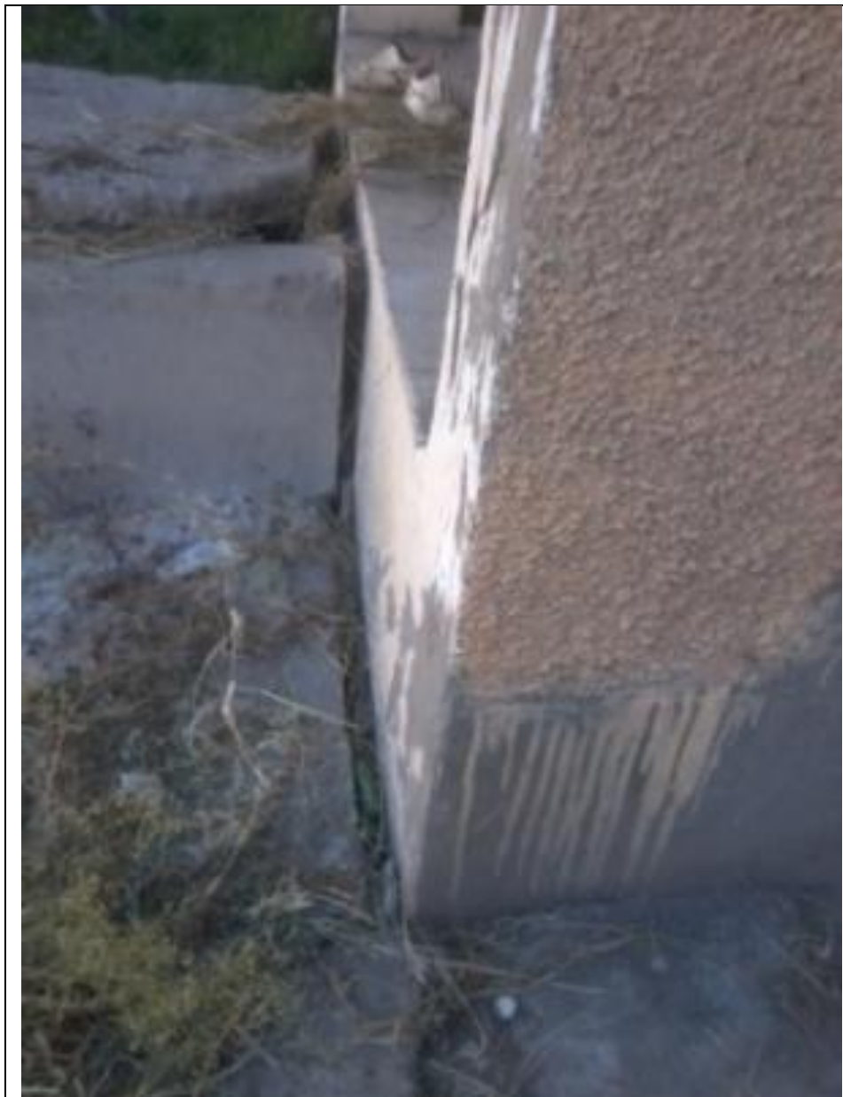
b)Cracks at its base
