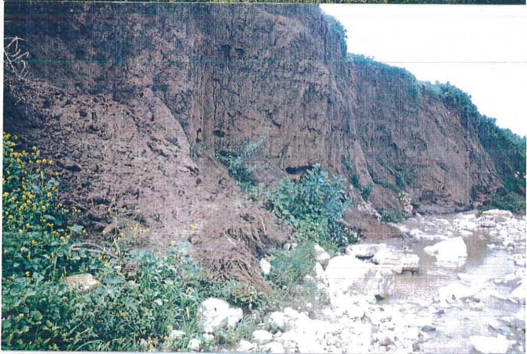
Photo 6. Deep and Wide Gully with its Collapse
