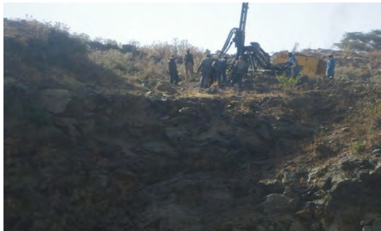
Figure 9: Drilling and blasting preparation to fragment the rocks in the study area
