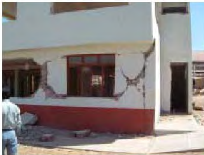
Fig. 4.2.4.2 Damaged CB wall and column. (Atico Earthquake - Peru 2001)
