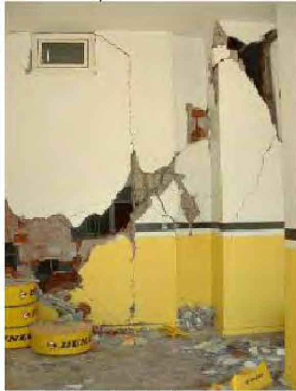
Fig. 4.2.4.3 Shear failures extending from the infills right across the column. (Bingol Earthquake - Turkey 2001)
