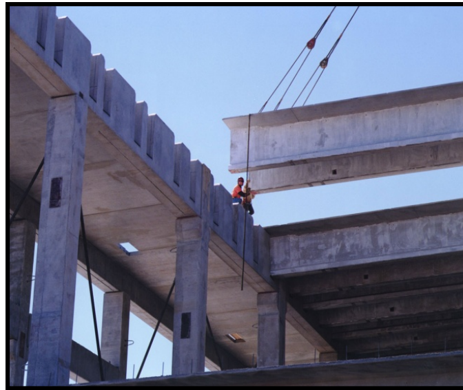
Figure 4.1: Layout of the T-section and the main girder beam [courtesy of white oak precast concrete semiconductor plant]
