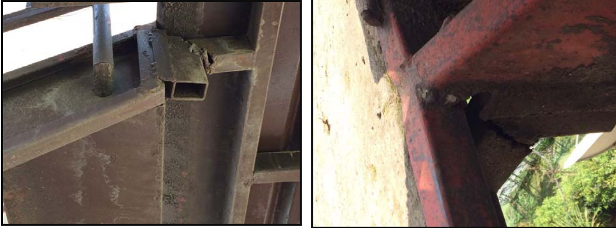
Figure 5.2: problems in stair connection of condominium site
