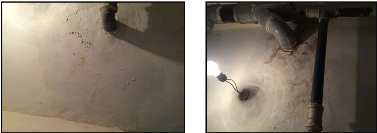
Figure 5.1: Problem in the current construction slabs
