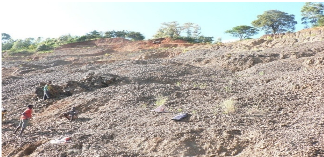
Figure 1. 3 Collapsed Retaining Wall and the Resulted Mud Flow
