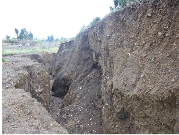
Figure2.4 Thick colluvial deposit collapsed along the road side
