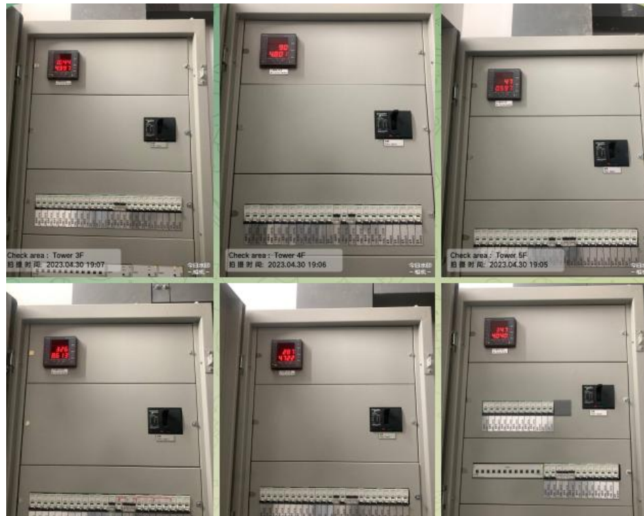
Figure 7-2: SDB based energy meters taken from different floors in CBE-HQ building
