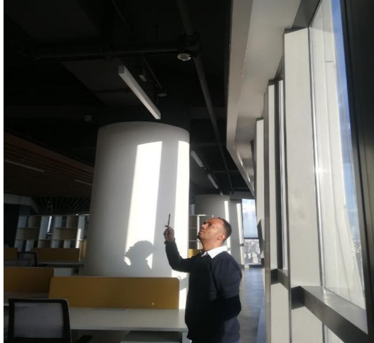
Figure 7-1: Daylight harvest sensors installed with the windows perimeter
