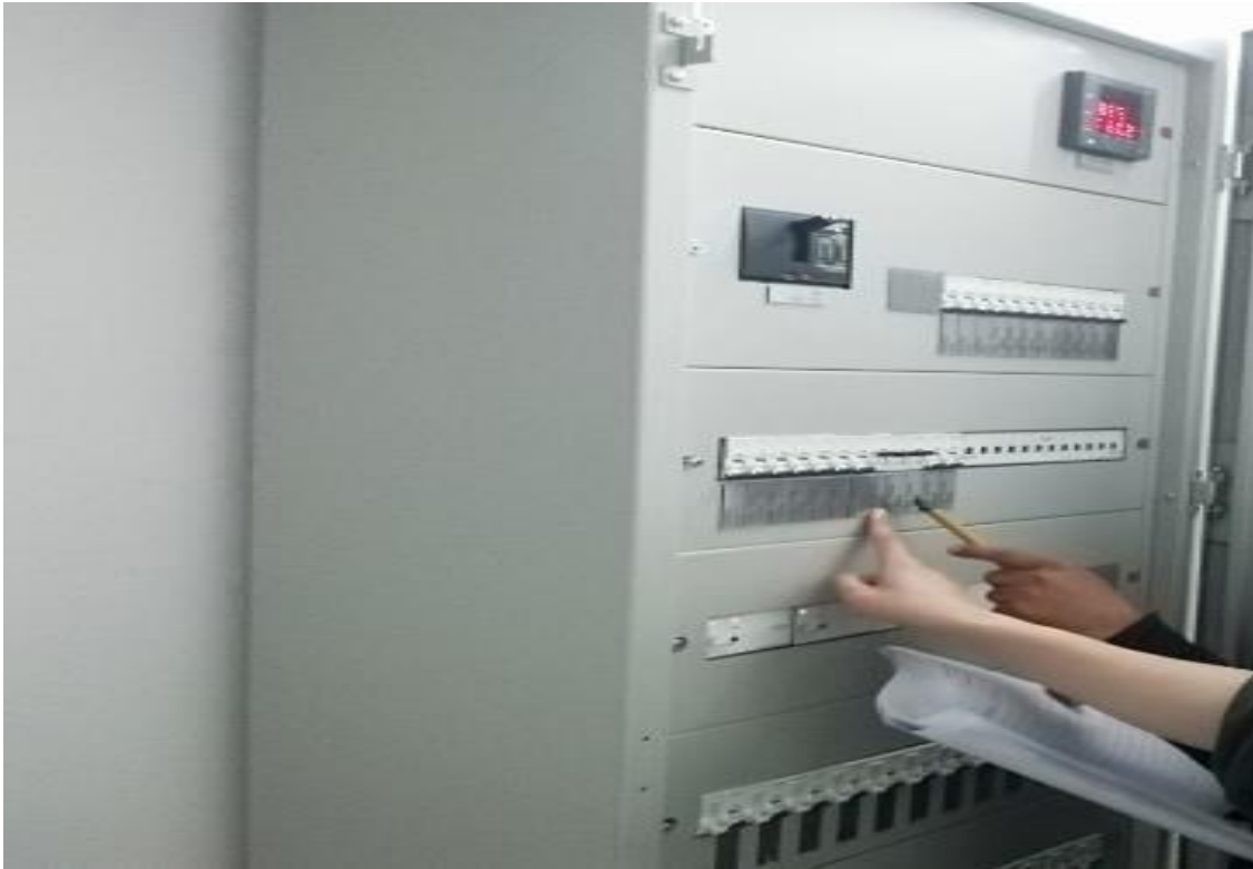
Figure 7-3: Identification and setting up of selected circuit breakers
