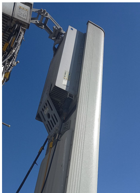
Figure 2.2: Ethio-Telecom 5G active antenna unit
