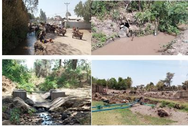
Figure 2-5 Breached structures, stone-regulated offtake, fully silted diversion weirs, and multi-use supply canal at Ketar and Arata Irrigation schemes. 9
