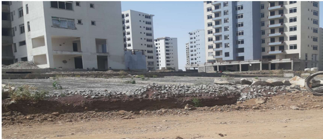
Figure 10: A figure showing partially demolished car parking due to lack of integration,
