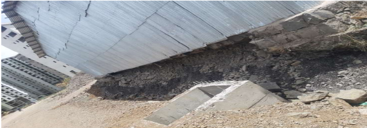
Figure 3: Damage by infrastructure supplying institutions at project site.
