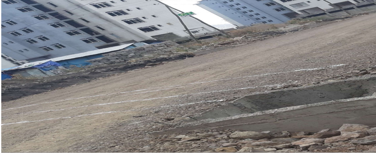
Figure 8: A figure showing the passing line of tele and electric utility under the road, According to an expert from the AACHDC's infrastructure department, this was the electrical and telecom utility line that would be excavated following the building of the main road at the project sites of the 20/80 housing provision. Infrastructure providing institutions might have easily avoided this by planning together at the start of any construction activity, or by examining the plans/designs of other infrastructure providing institutions if they were developing separately.
