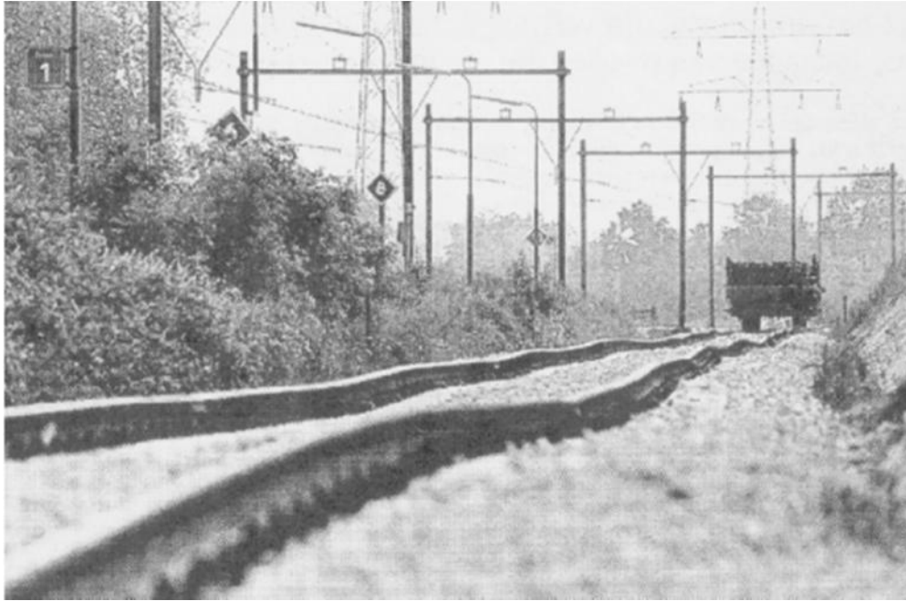
Figure 2-2 Deterioration of a railway track
