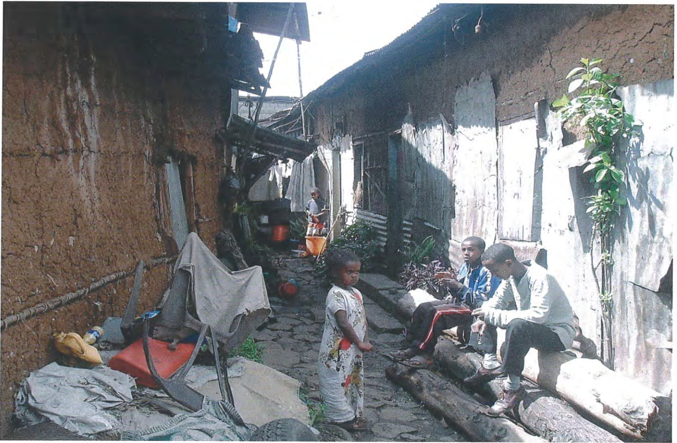
Figure 3.4: The Condition of Publicly Own Kebele Row Houses Source: Field survey around former kebele 34, 2010
