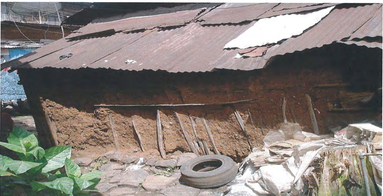
Figure 3.5: The Condition of Publicly Own Kebele Row Houses. Source: Field survey around Amanuel, 2010
