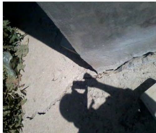
Fig. 1.2 Crack on office building of the project
