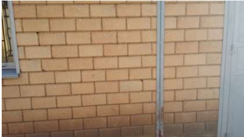
Figure 2-5: Wall made from interlocking CEBs in Selam Technical and Vocational Center, Addis Ababa
