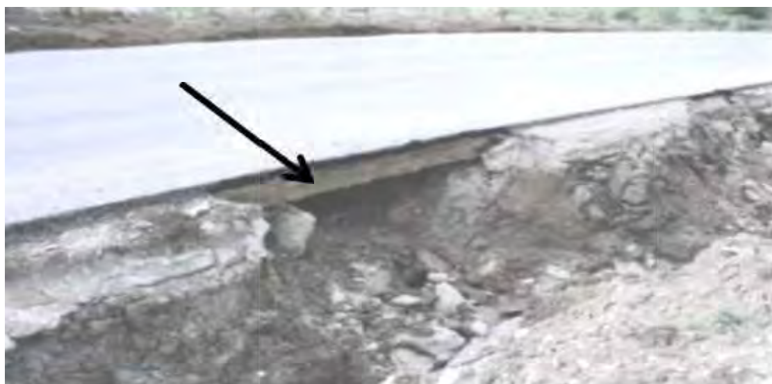
Fig.3.4 Lime-stabilized layer (see arrow) bridging an erosion failure illustrates strength.[14]
