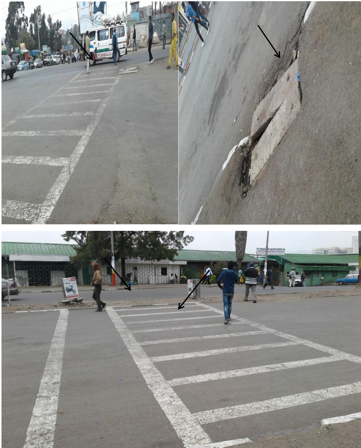
Figure 36.Photo.Interrupted pedestrian cross marking, poor drainage
