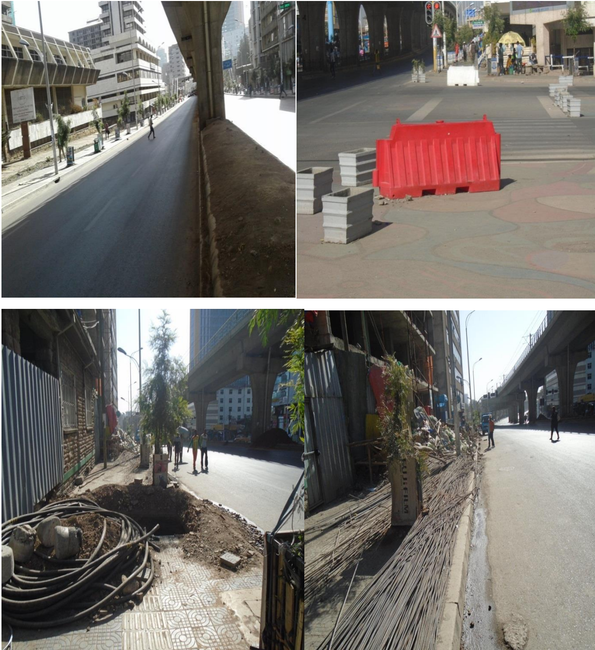
Figure 6. Photo. Faded longitudinal and pedestrian cross markings, unprotected utility line burrow, construction materials on walkway.
