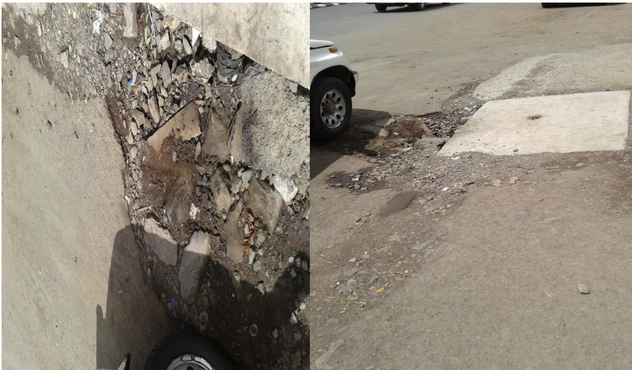
Figure 27.Photo.Excavated material on walkway, blocked road side drain
