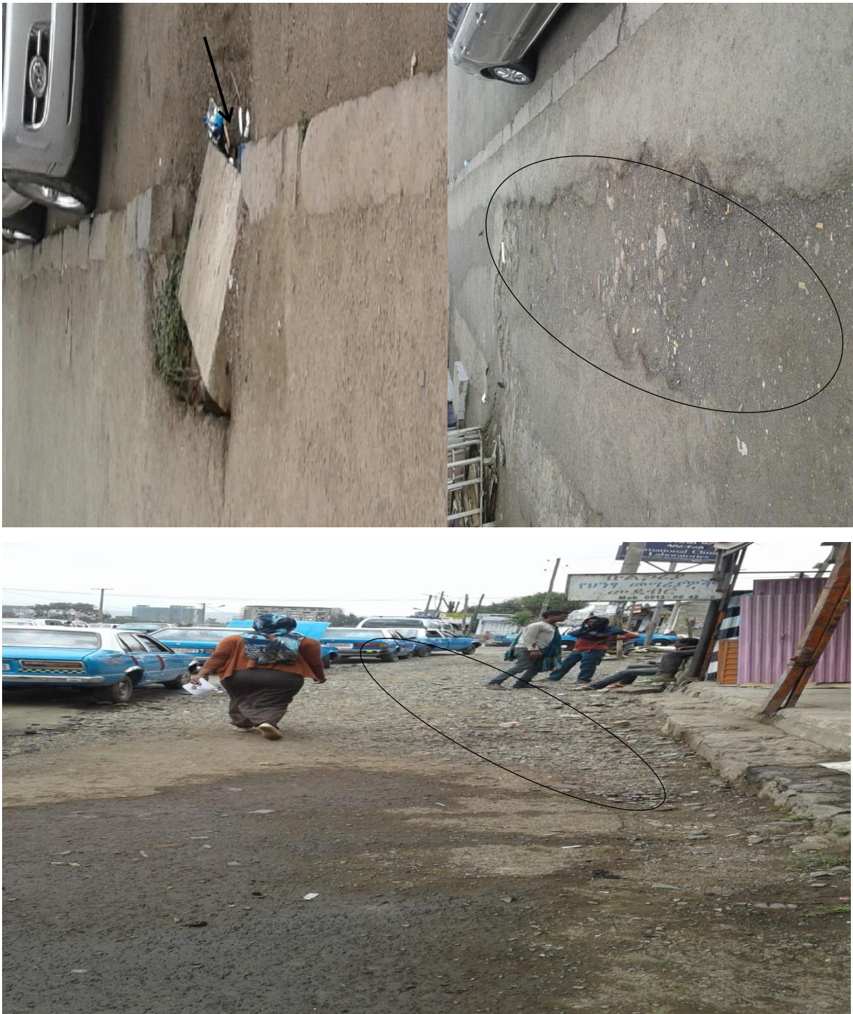
Figure 30.Photo.Deteriorated walk way, blocked inlet
