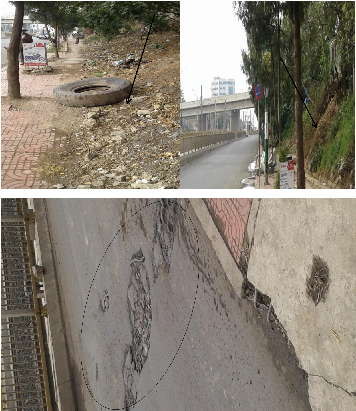
Figure 39. Photo. Trashes and vegetation reduced walk way width, Pavement surface deterioration
