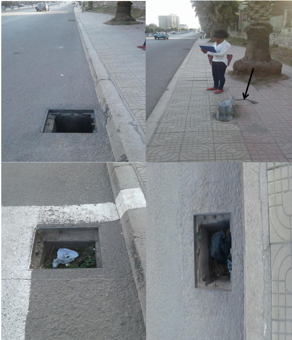
Figure 19. Photo. Uncovered ditch filled with dirt, damaged lighting
