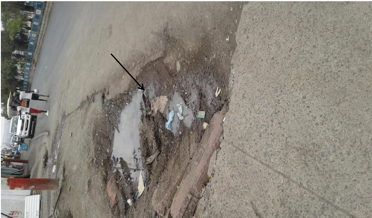
Figure 29. Photo. Pavement crack and blocked roadside drainage inlet
