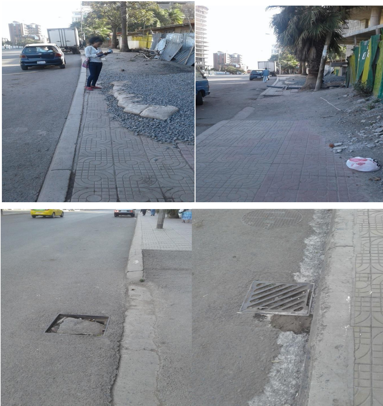
Figure 9. Photo. Construction material on the walkway, blocked inlet, improper inlet cover
