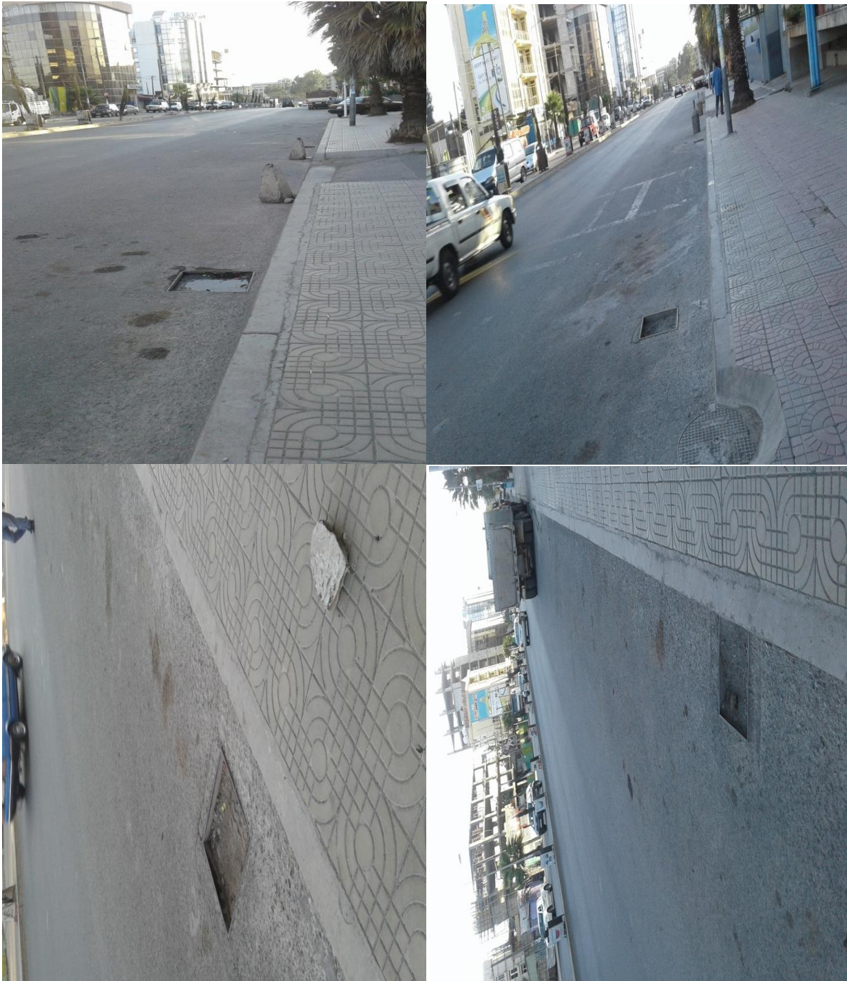
Figure 17. Photo. Uncovered and blocked road side drainage inlets filled with dirt
