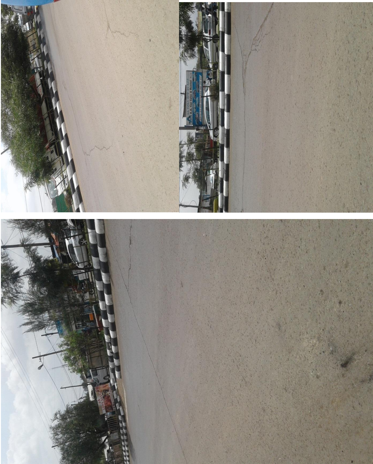
Figure 28. Photo. Longitudinal and transverse pavement crack
