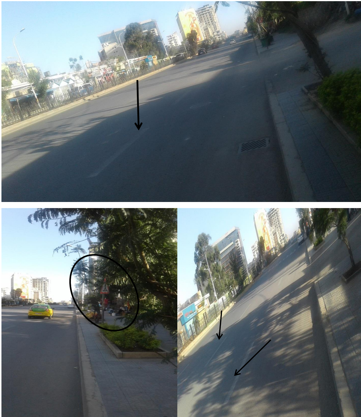
Figure 22.Photo.Faded road marking, road side vegetation obstruct visibility of traffic sign
