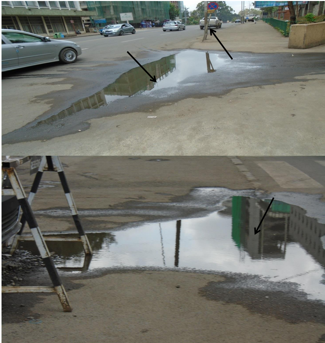
Figure 1. Photo. Water ponding on the walk way & pavement edge, damaged traffic sign & Lighting pole
