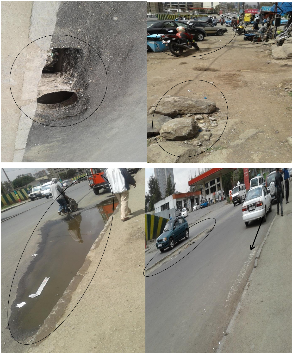
Figure 32. Photo. Uncovered ditch, ponding of water on the pavement surface, faded pedestrian cross marking, damaged median, obstructed walkway
