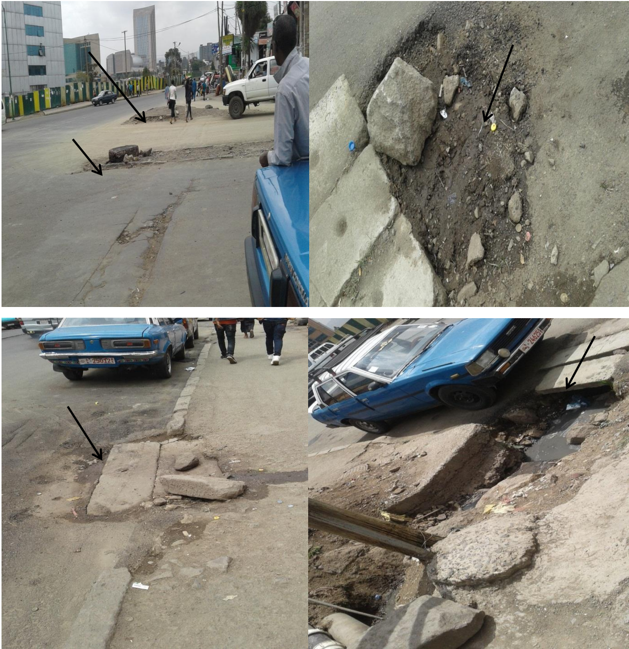
Figure 31. Photo. Deteriorated Island, blocked poor drainage
