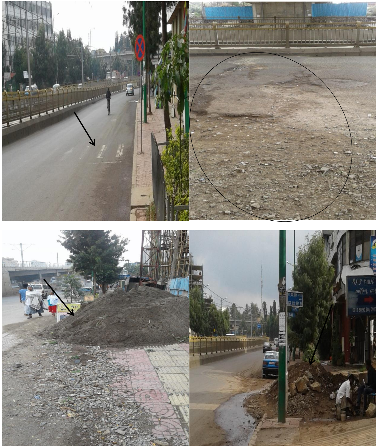
Figure 43. Photo. Unremoved pedestrian cross marking, Deteriorated pavement surface, dumped construction material on walkway, excavated material on walk way
