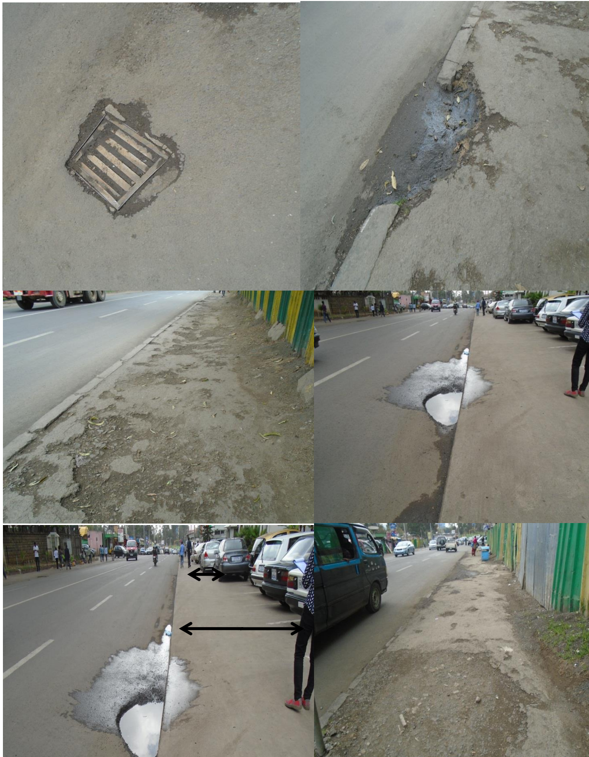
Figure 2. Photo. Blocked road side drainage, deteriorated walks way and walk way reduced by parked vehicle.
