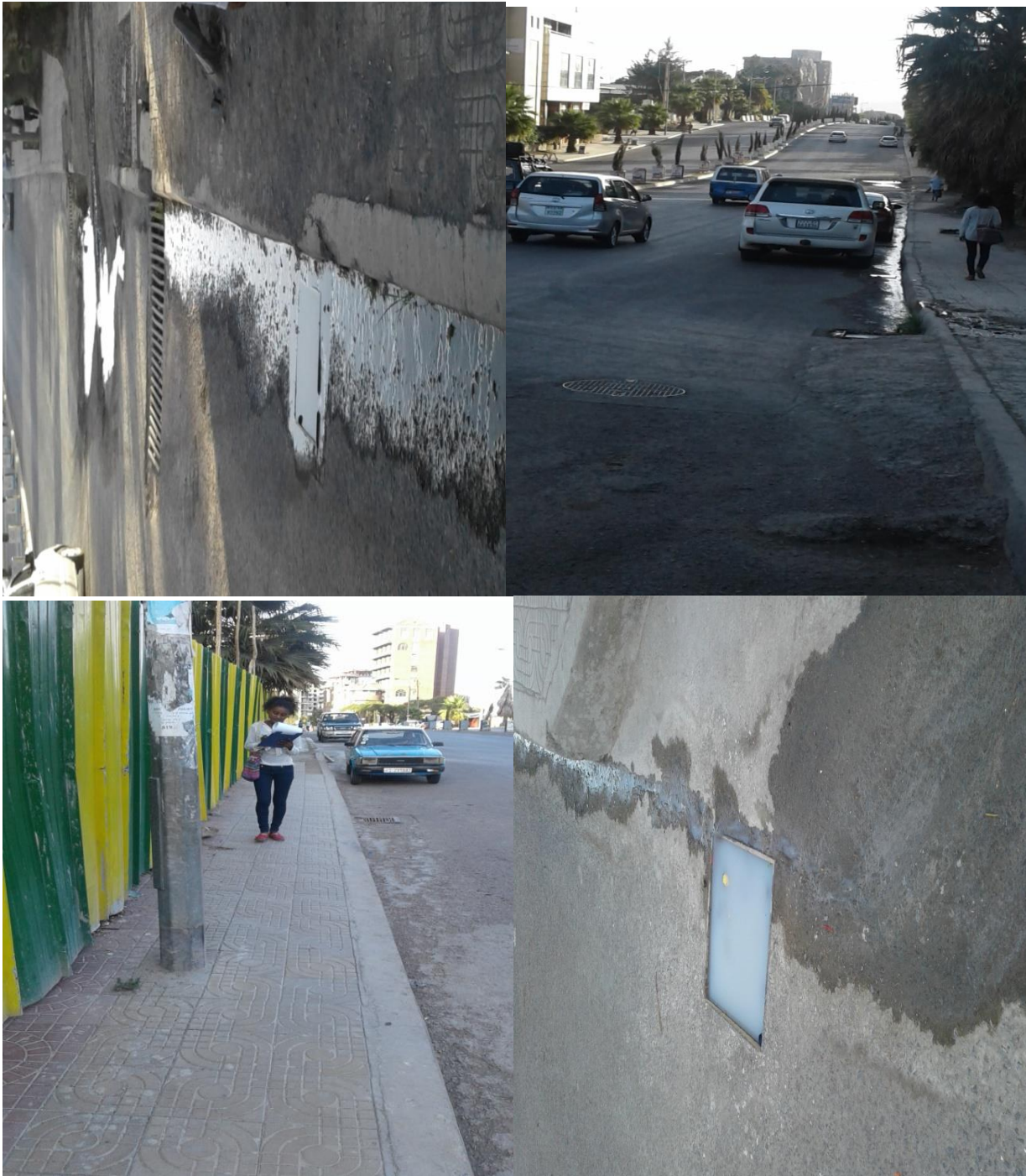
Figure 20. Photo. Ponding water on the pavement surface due to poor drainage, steep vertical alignment, construction fence reduce walkway width
