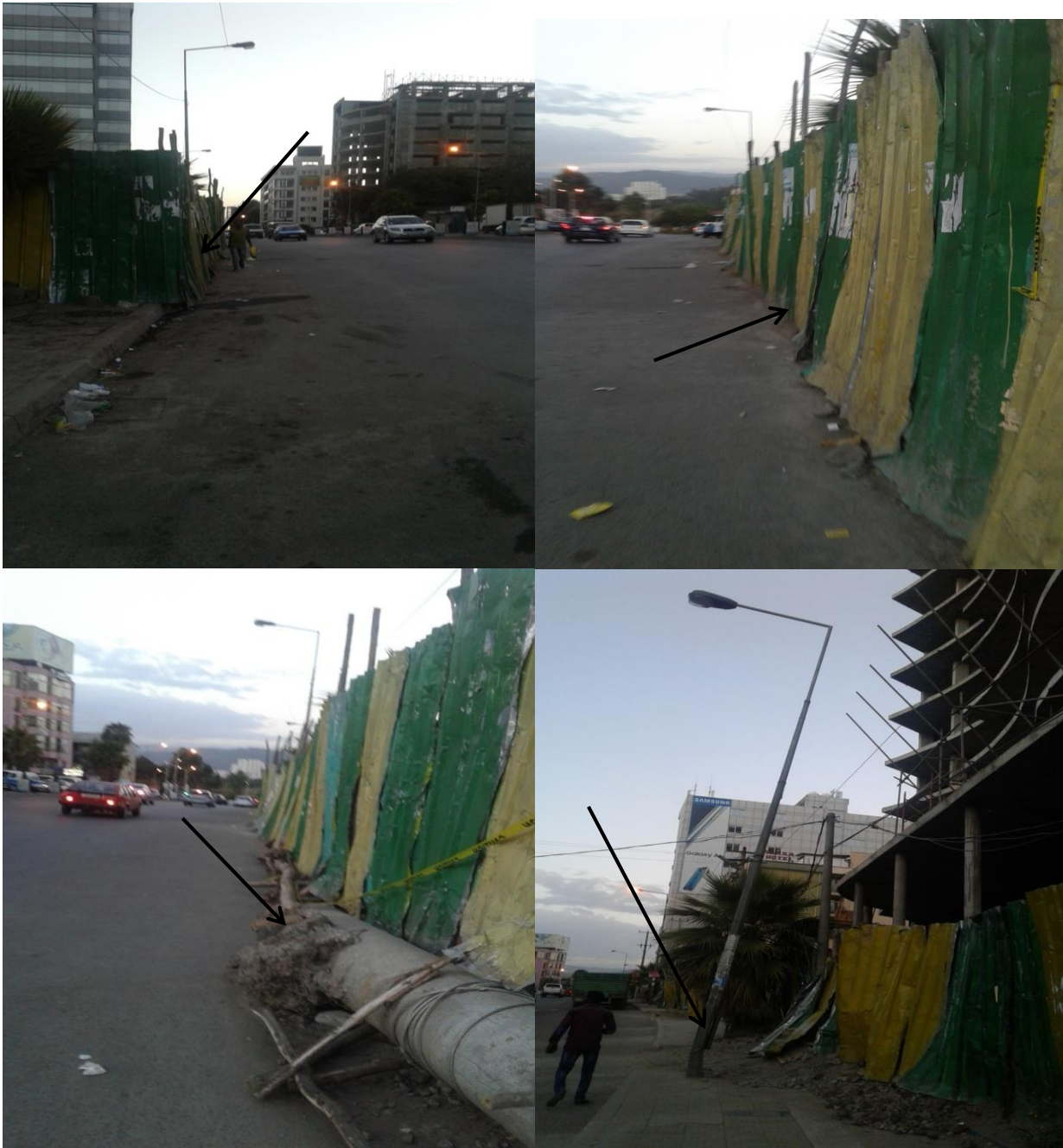
Figure 10. Photo. Construction fence block the walk way and obstruct both pedestrian and vehicle movement, damaged lighting
