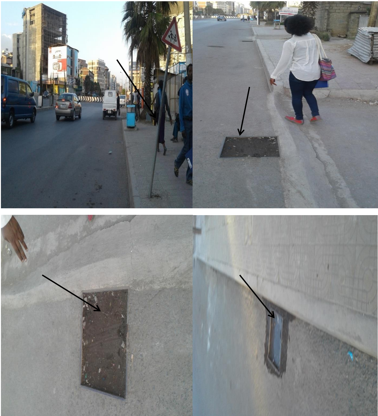
Figure 14. Photo. Damaged traffic sign, blocked ditches.
