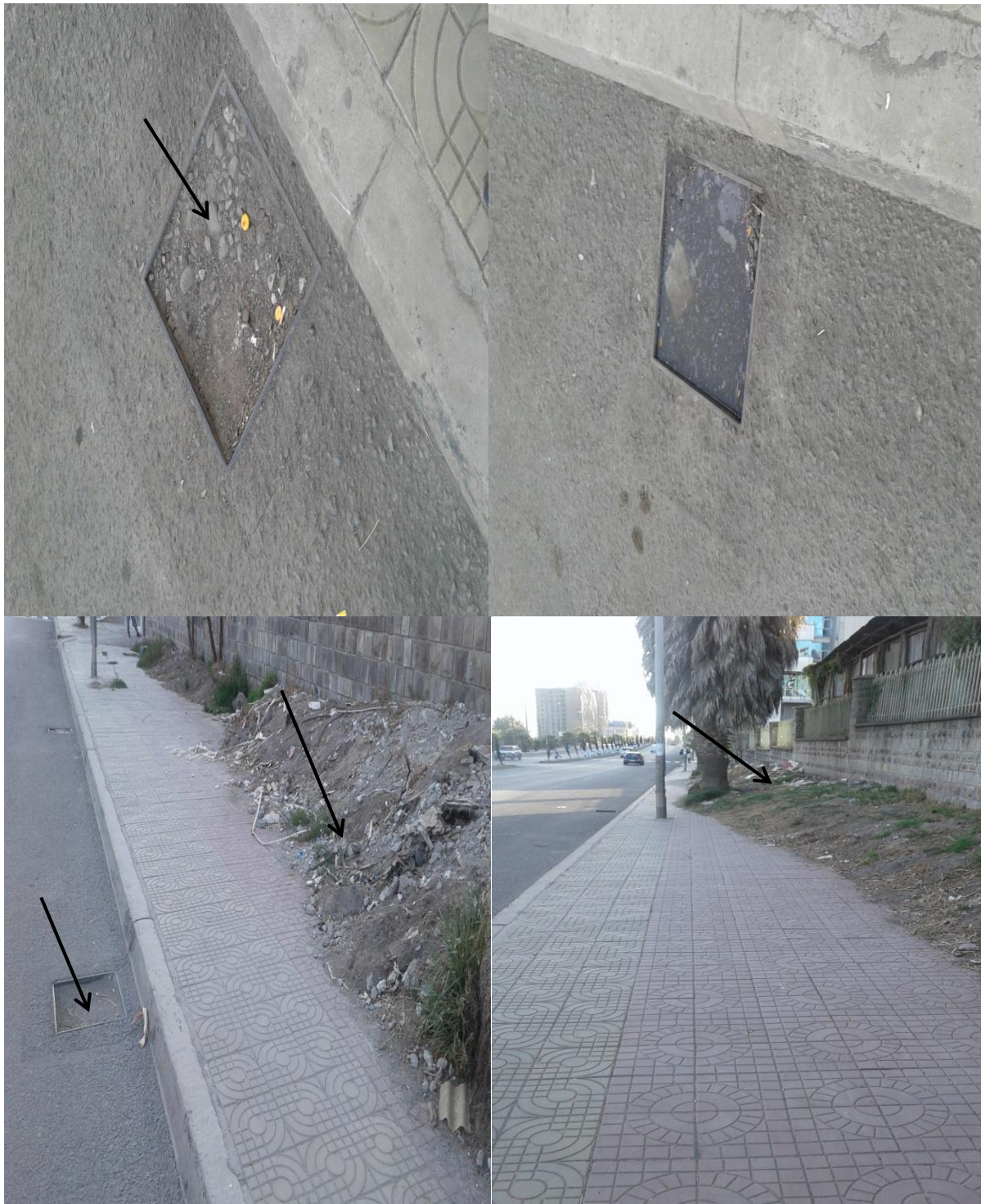
Figure 18. Photo. Blocked inlets, trashes on walkway
